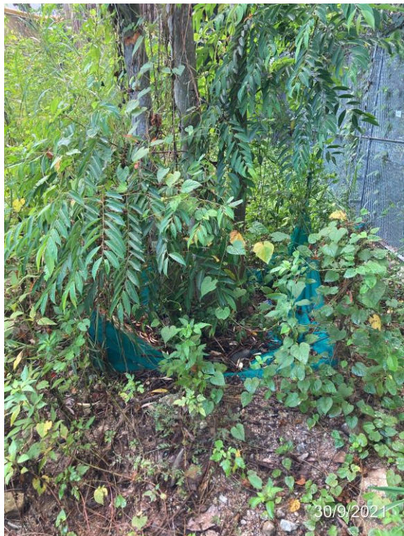
Photo 10. Collapsed fencing to be rectified. The climbers and weeds shall be cleared.
