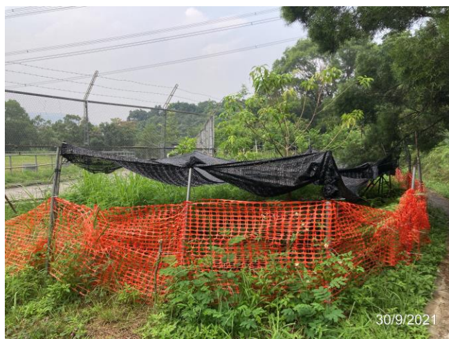
Photo 2. Collapsed fencing has been rectified
