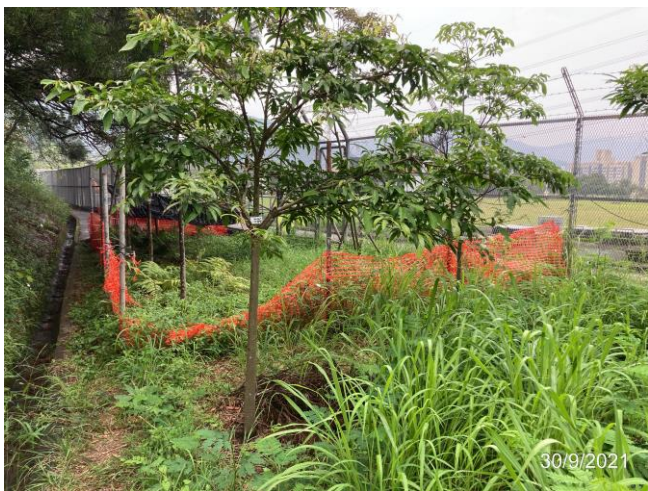
Photo 5. Collapsed fencing to be rectified
