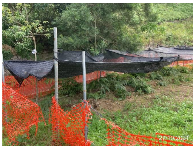
Photo 2. Broken fencing to be rectified
