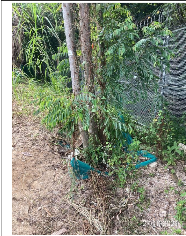
Photo 10. Collapsed fencing to be rectified. The climbers and weeds have been cleared.
