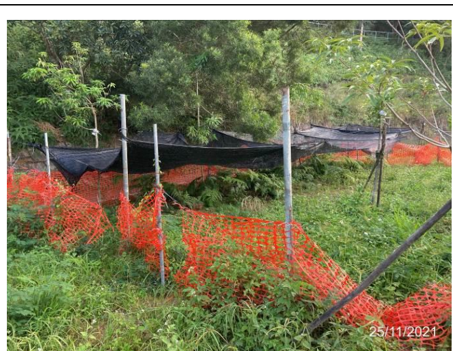
Photo 2. Broken fencing to be rectified
