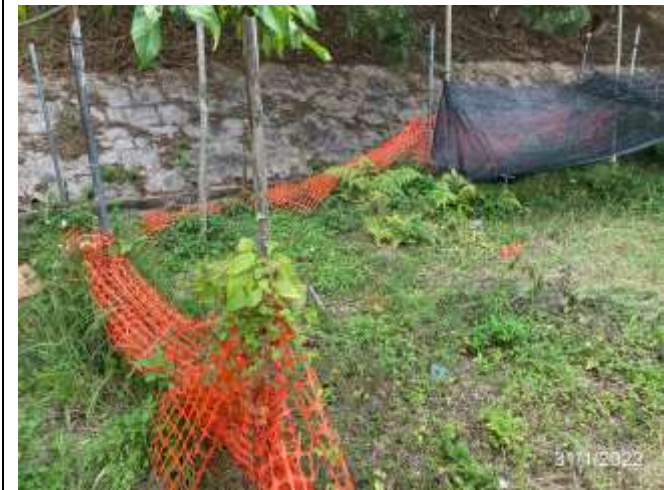
Photo 3. Broken fencing to be rectified
