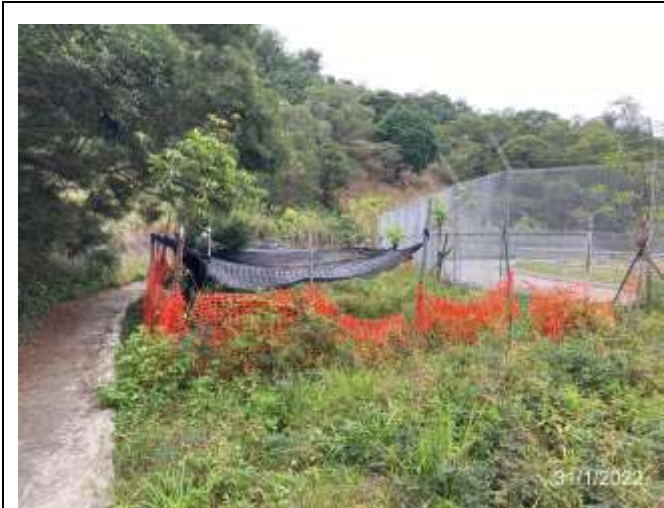
Photo 1. Broken fencing to be rectified
