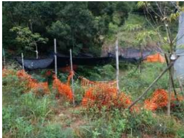
Photo 2. Broken fencing to be rectified
