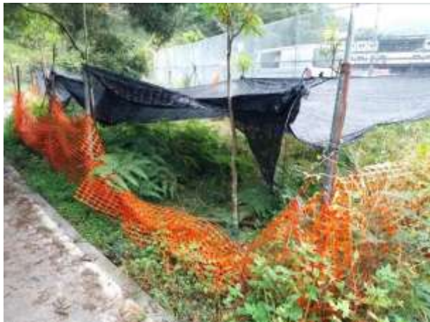
Photo 1. Broken fencing to be rectified
