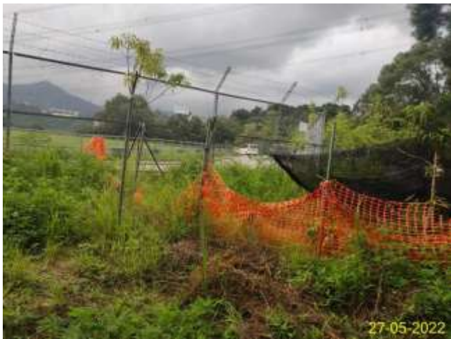
Photo 3. Broken fencing to be rectified
