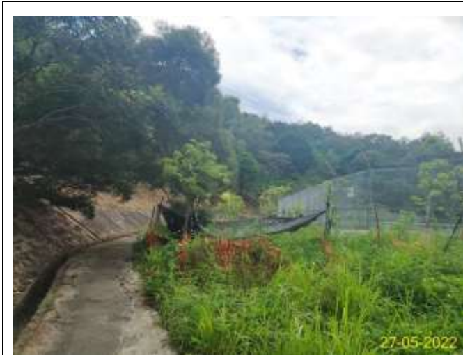
Photo 1. Broken fencing to be rectified
