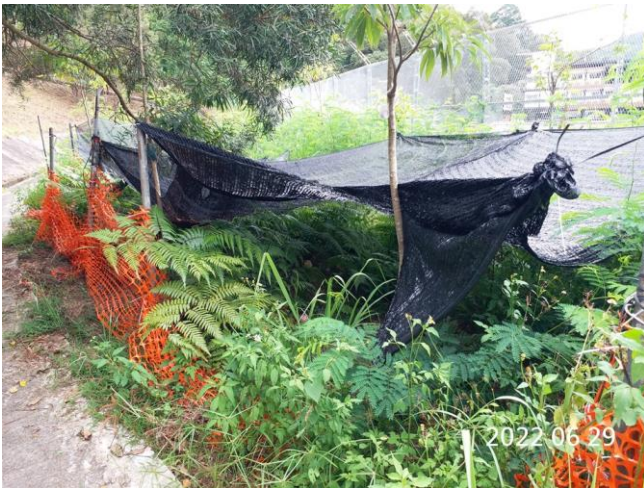
Photo 1. Broken fencing to be rectified
