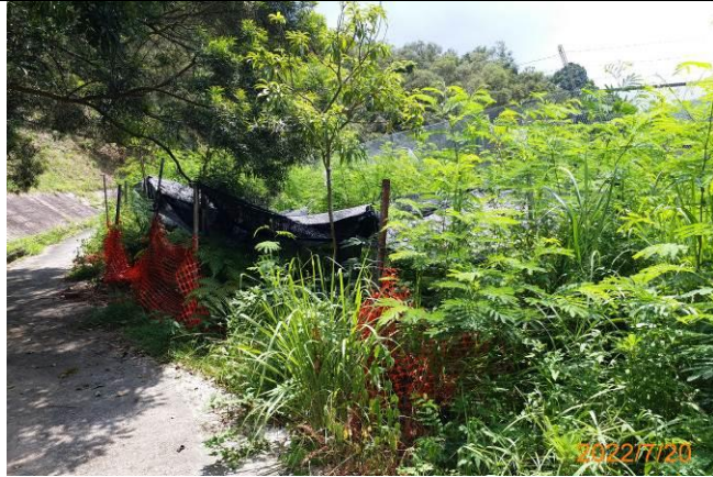
Photo 1. Broken orange fencing to be rectified
