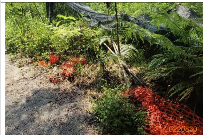
Photo 3. Broken orange fencing to be rectified
