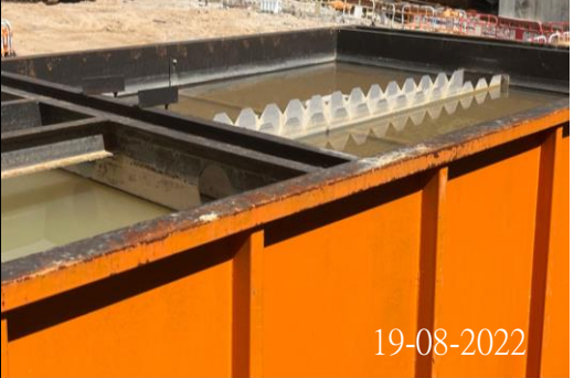
Photo 5 (Water quality of water treatment tank at 6/WSD)
