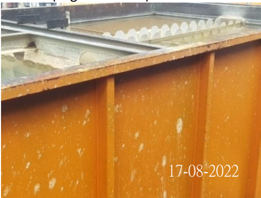
Photo 6 (Water quality of water treatment tank at 6/WSD)
