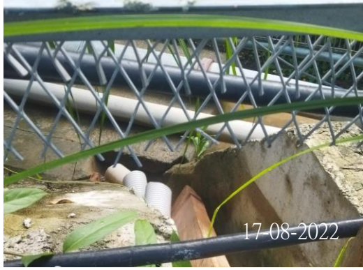
Photo 7 (Discharge point at 6/WSD)
