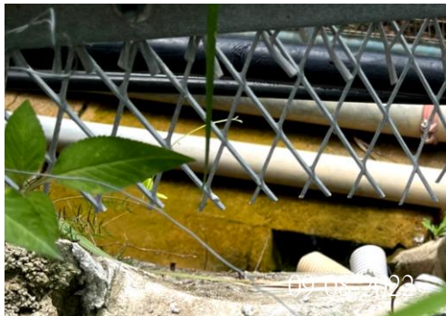
Photo 7 (Discharge point at 6/WSD)
