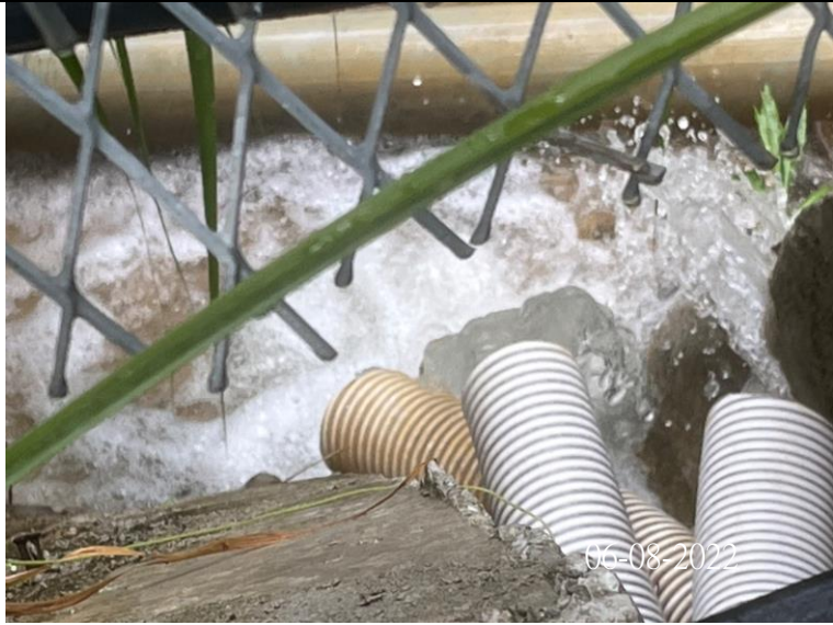
Photo 3 (Discharge point at 6/WSD)
