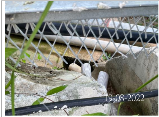
Photo 6 (Discharge point at 6/WSD)
