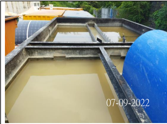
Photo 3 (Water quality of water treatment tank at 6/WSD)
