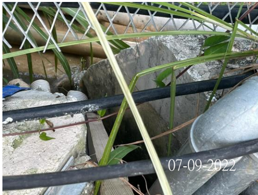
Photo 4 (Discharge point at 6/WSD)
