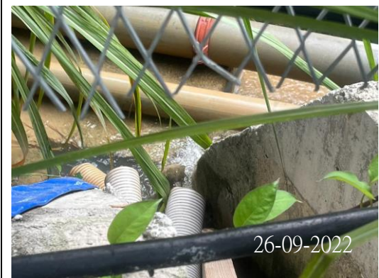
Photo 3 (Discharge point at 6/WSD)
