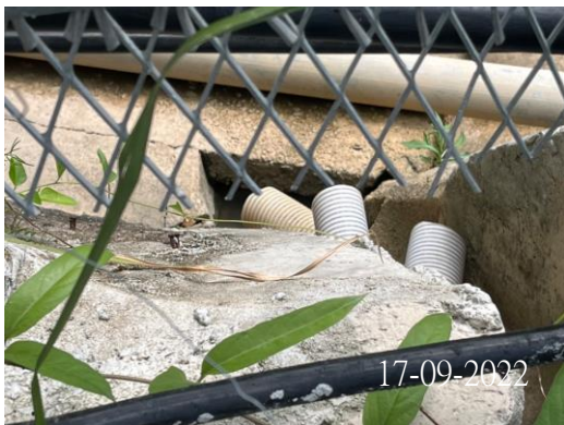
Photo 3 (Discharge point at 6/WSD)
