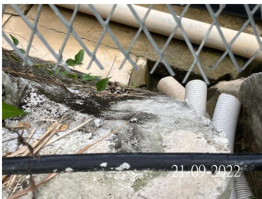
Photo 3 (Discharge point at 6/WSD)
