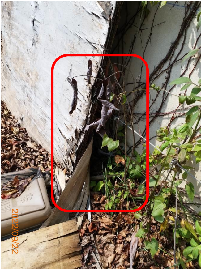
Photo 10. Dead Desmos chinensis . Construction materials shall be taken away from the planting zone to avoid soil compaction, and potential disturbance to the plant before re-planting.
