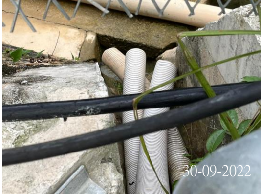
Photo 8 (Discharge point at 6/WSD)
