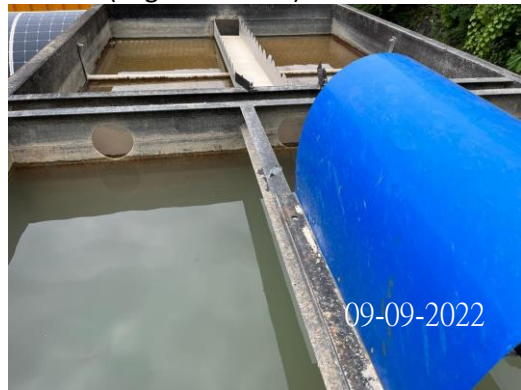
Photo 4 (Water quality of water treatment tank at 6/WSD)
