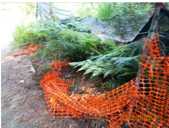
Photo 1. Broken orange fencing to be rectified
