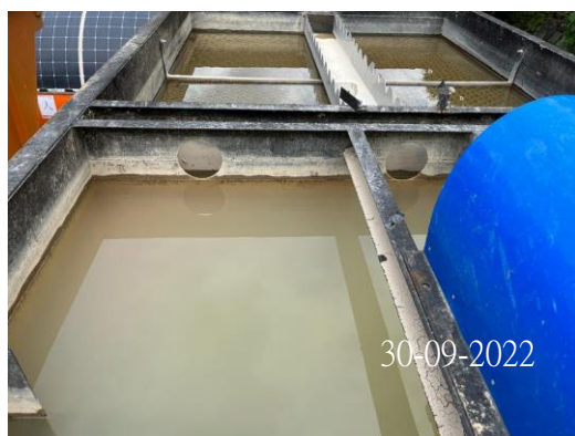
Photo 7 (Water quality of water treatment tank at 6/WSD)
