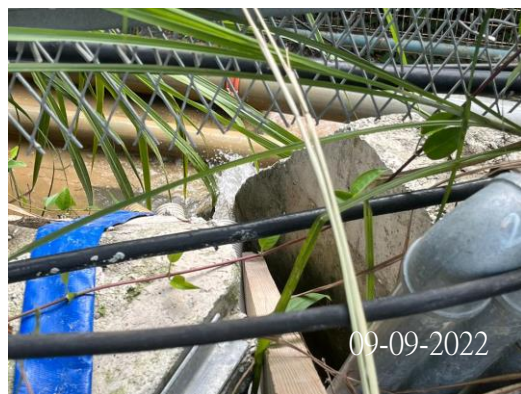
Photo 5 (Discharge point at 6/WSD)
