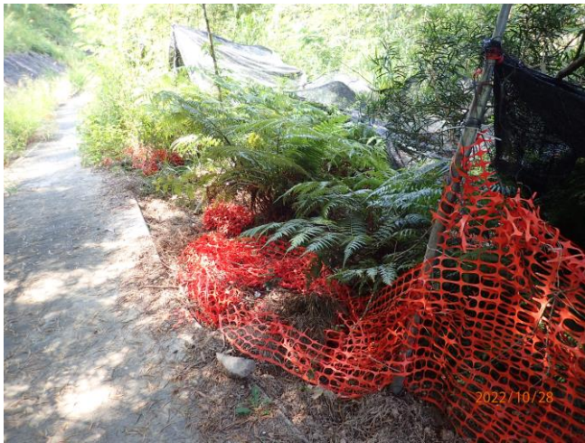
Photo 1. Broken orange fencing to be rectified
