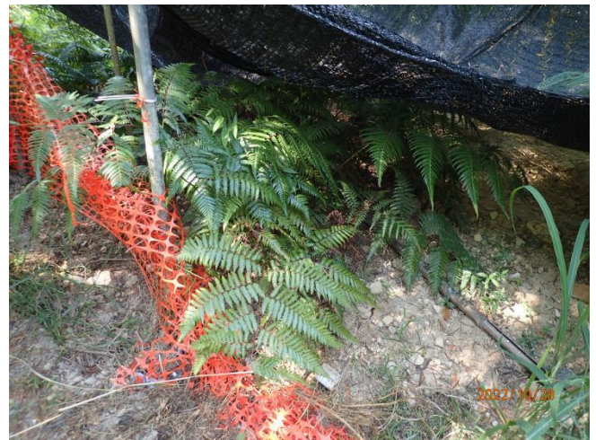
Photo 4. Broken orange fencing to be rectified
