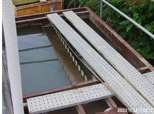
Photo 4 (Water quality of water treatment tank at 1/WSD)
