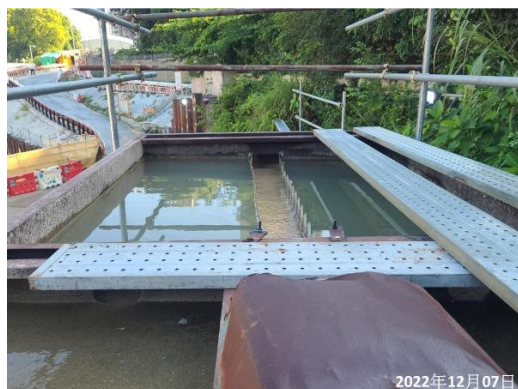
Photo 5 (Water quality of water treatment tank at 1/WSD)
