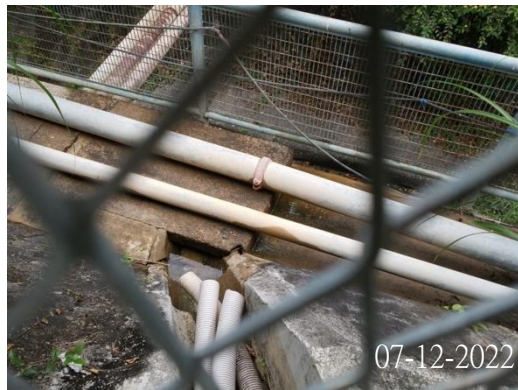
Photo 4 (Discharge point at 6/WSD)
