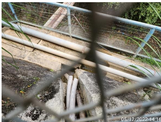
Photo 3 (Discharge point at 6/WSD)
