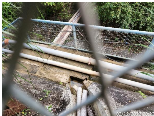
Photo 3 (Discharge point at 6/WSD)
