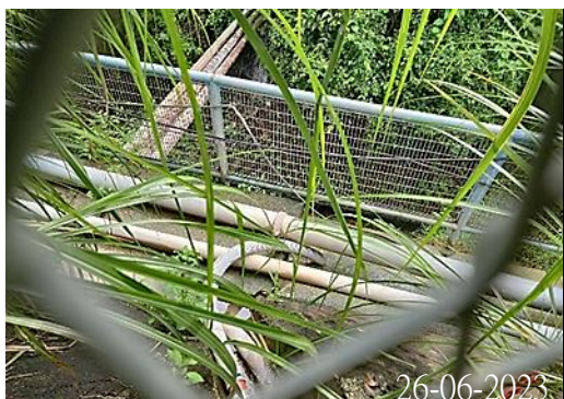
Photo 3 (Discharge point at 6/WSD)
