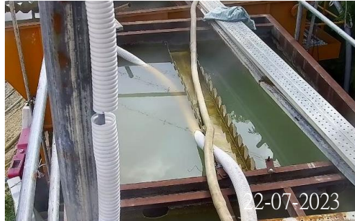
Photo 4 (Water quality of water treatment tank at 1/WSD)
