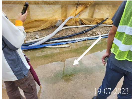
Photo 5 (Water accumulation on the road surface on 1/WSD)
