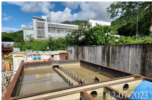
Photo 2 (Water quality of water treatment tank at 6/WSD)
