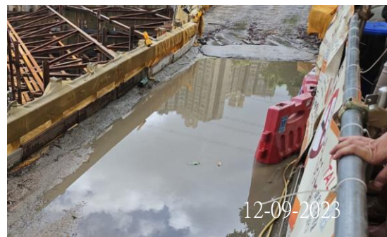
Photo 6 ( Water accumulation on the site area at 1/WSD)
