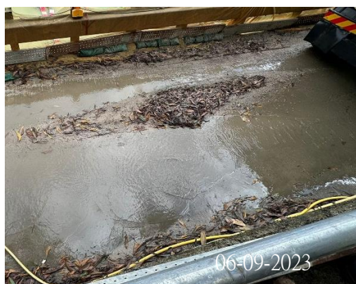
Photo 5 (Water accumulation on the M1 to M5 at 1/WSD)
