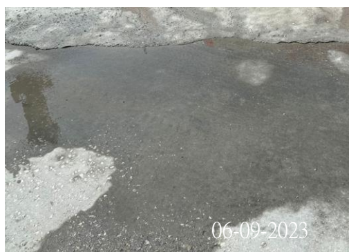
Photo 6 (Water accumulation on the site area at 6/WSD)
