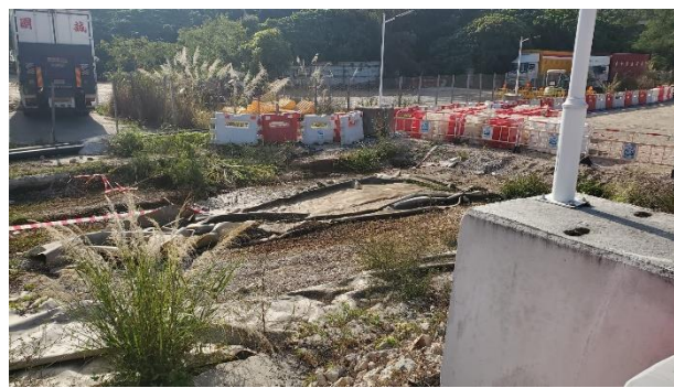
All wastewater / surface runoff was collected and diverted to sump pit. Direct effluent discharge was not allowed to be discharged from the site. No discharge of wastewater was observed during site investigation.
