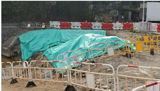
Stockpile of dusty materials was covered properly to avoid generation of muddy runoff.
