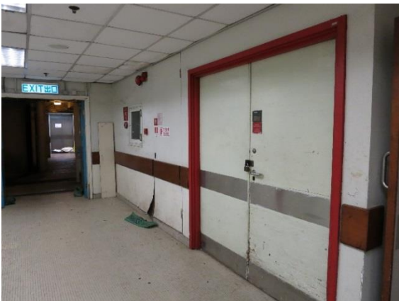
Figure 3.15 Entry of the Incinerator Room
