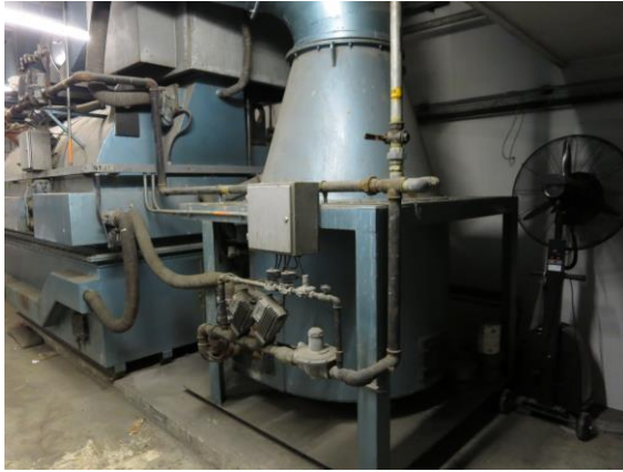
Figure 3.5 Secondary Combustion Chamber of Incinerator No.1
