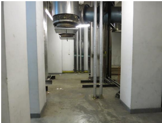
Figure 3.7 View of Incinerator Room 1
