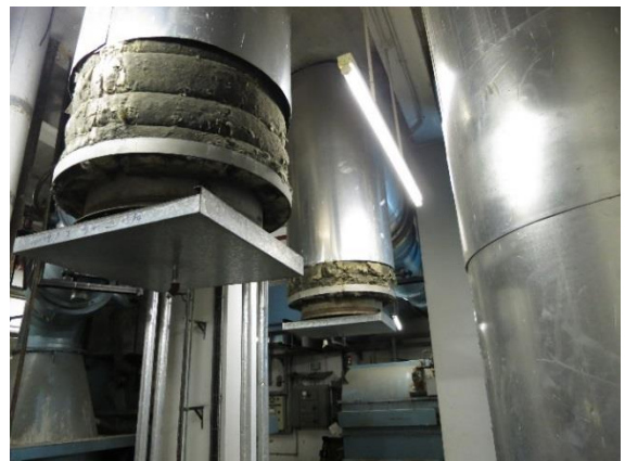
Figure 3.10 Chimneys to be sealed up
