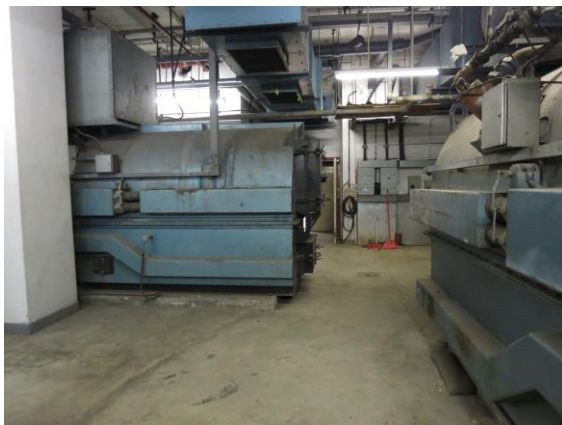
Figure 3.9 Overview of the Incinerator Room
