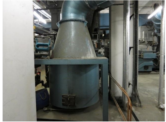
Figure 3.6 Secondary Combustion Chamber of Incinerator No.2
