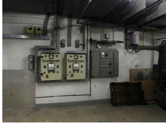
Figure 3.12 Control panels for incinerators, DDC control, exhaust fan for LG501D compressor/vacuum equipment room and TPN for boiler isolation
