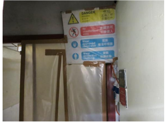
Figure 3.4 Environmental and Safety Notices and Warning Signs were posted in the entry of the three-compartment decontamination unit
