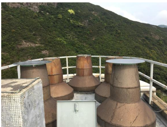
Figure 3.13 Sealed Chimneys at the Rooftop
