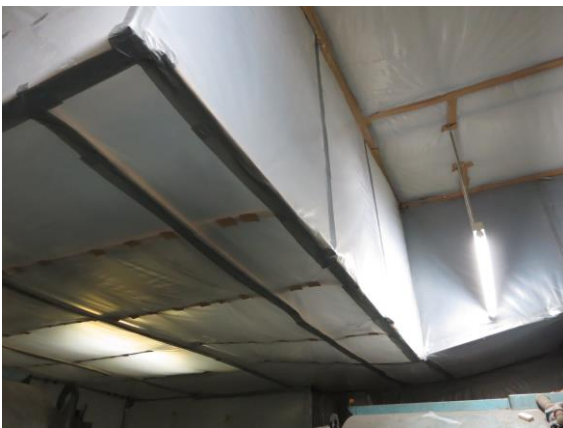
Figure 3.1 View of Incinerator Room
