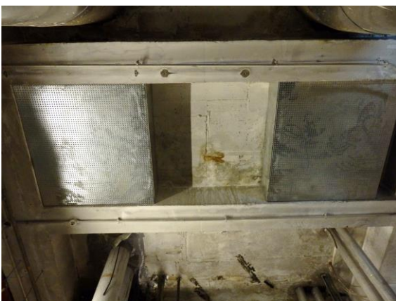
Figure 3.7 Chimneys were sealed up
