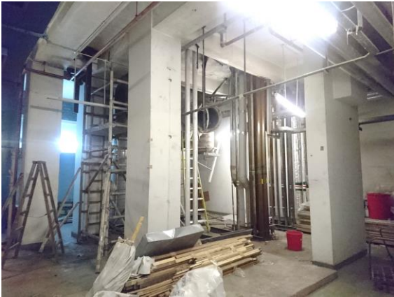
Figure 3.4 View of Incinerator Room
