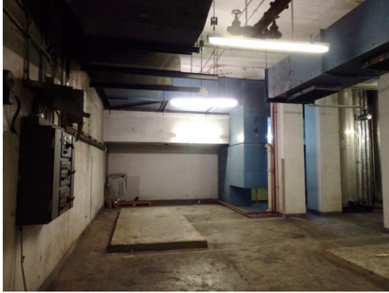
Figure 3.9 View of Incinerator Room
