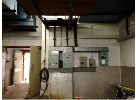
Figure 3.10 Fused link boxes to be retained
