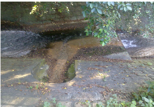
Muddy stain was observed at the exit of the closed channel at upstream near Shing Mun Lane.
