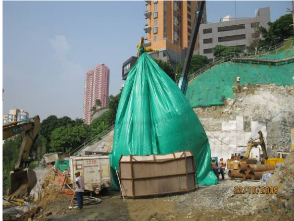
Photo no. 2 Movable barrier for Drilling rig
