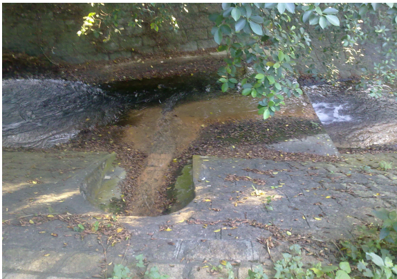
Muddy stain was observed at the exit of the closed channel at upstream near Shing Mun Lane.
