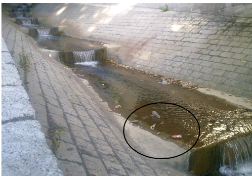
Rubbish was observed at I-1-C
