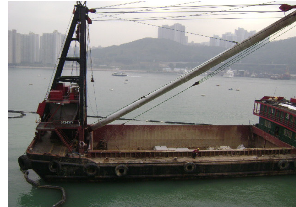
Photographic record for exceedance of Dissolved Oxygen (marine surface) recorded at O-1(FT) on 07-Dec-11
