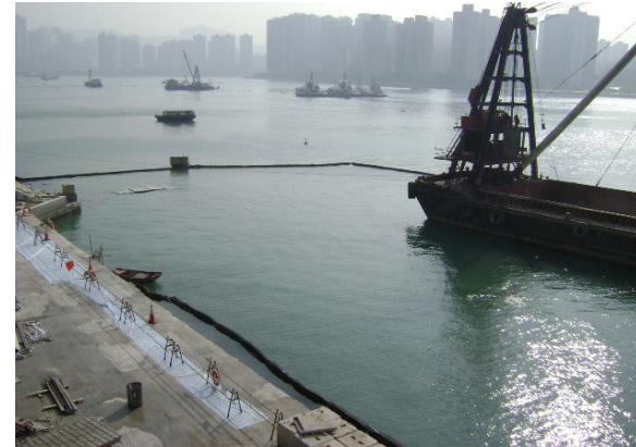
Photographic record for exceedance of Dissolved Oxygen (marine surface) recorded at O-1(FT) on 16-Dec-11
