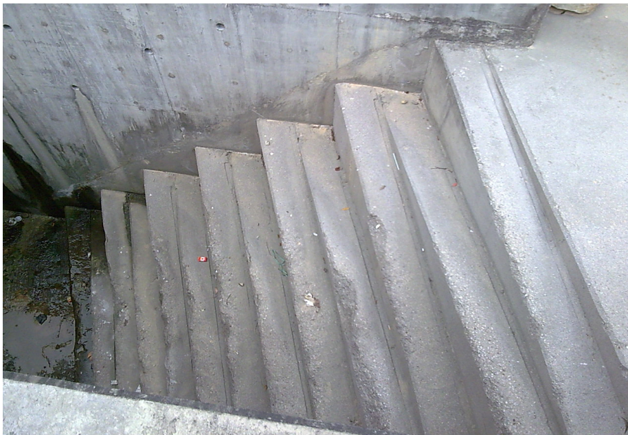
(8) The sloped Step at Wildlife Ramp (A)
