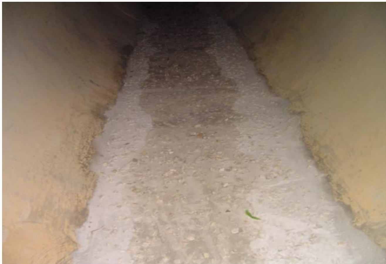
(4) Opening of Wildlife Tunnel with Wildlife Ramp (B)
