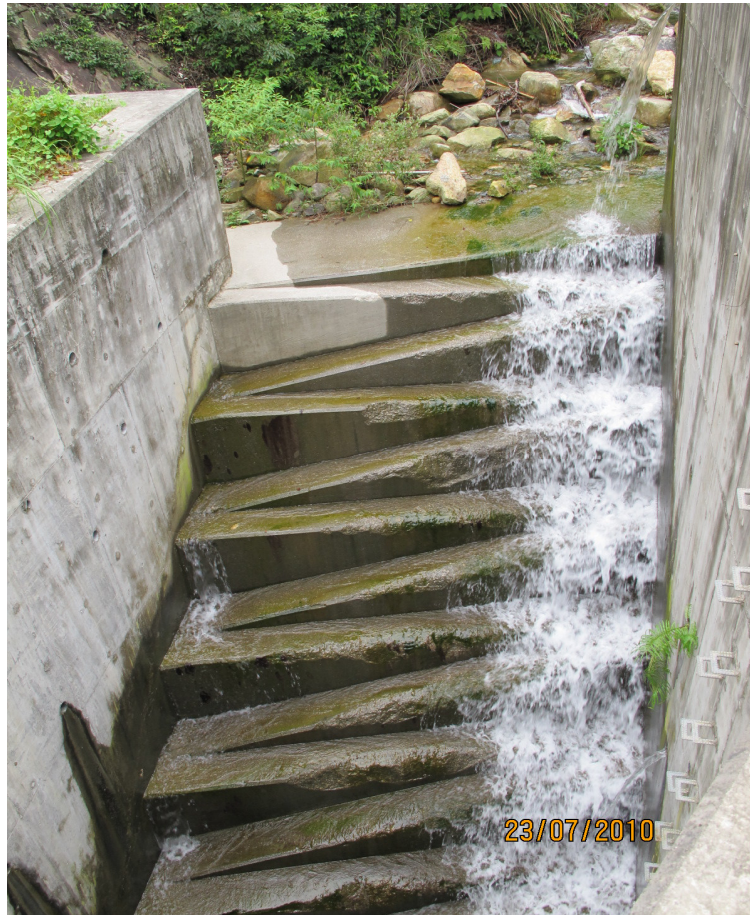
(7) The sloped Step at Wildlife Ramp (A)
