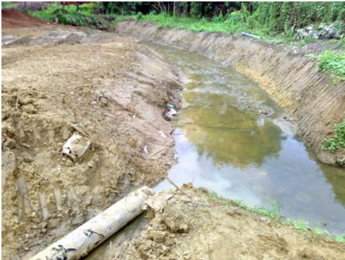
Obs 1 – Some silty water seepage into the stream was observed (CH155) during the site inspection, the Contractor was reminded to confine the wastewater/runoff and divert to the sedimentation system prior to discharge.
