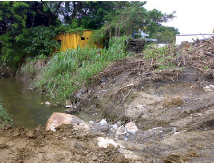
C&D wastes/excavated soil accumulated next to stream edge at CH200 had been remove. (ref: KT15-160807).
