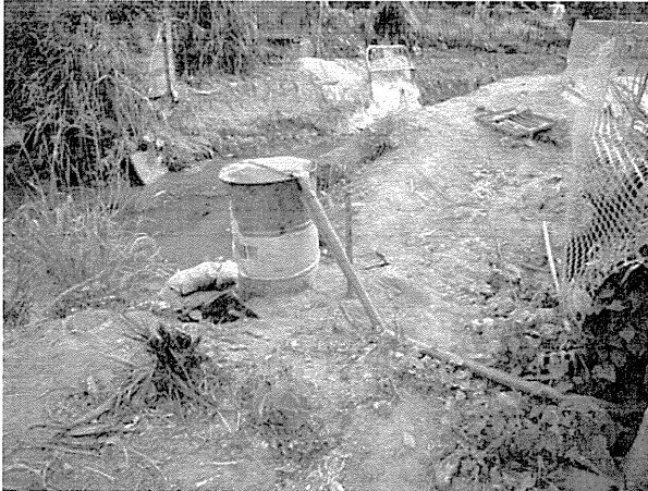
Sedimentation tank was provided for the discharge at CH-200.
