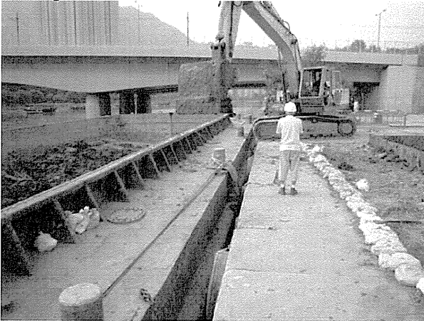
Contractor was reminded to provide cover the gap between barge and pier to avoid splashing of material into the sea.
