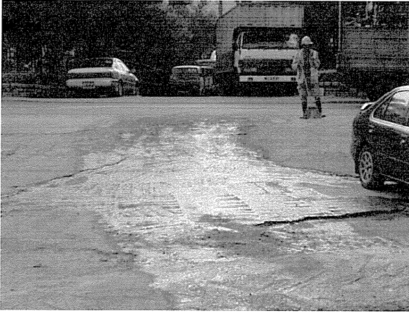
The contractor was reminded to repair the concrete bare ground in front of the wheel washing bay to reduce the amount of mud and dust deposited outside the site of public road at CH-470.
