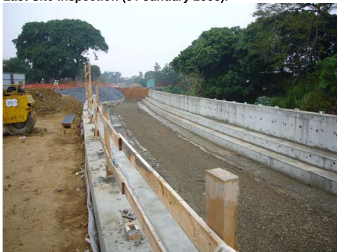
Stagnant water at CH 270 was cleared
