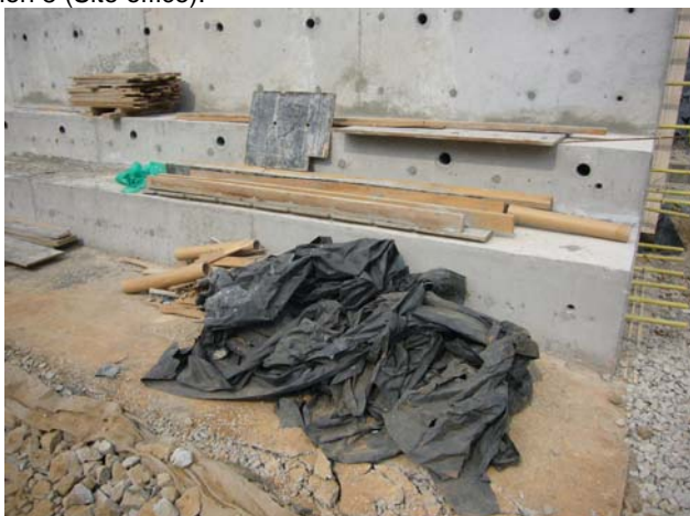
Some C&D waste scattered on-site was observed at CH 180, the Contractor was reminded to tight up the working area.
