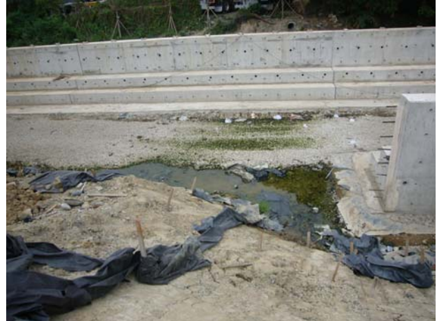
Stagnant water was accumulated at CH 200 & 504, the Contractor was reminded to clean to prevent mosquito breeding. (On- going)
