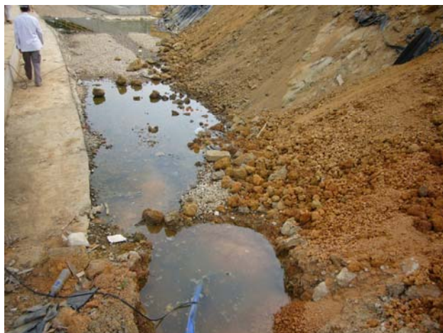
Stagnant water was accumulated at CH 200, the Contractor was reminded to clean to prevent mosquito breeding.
