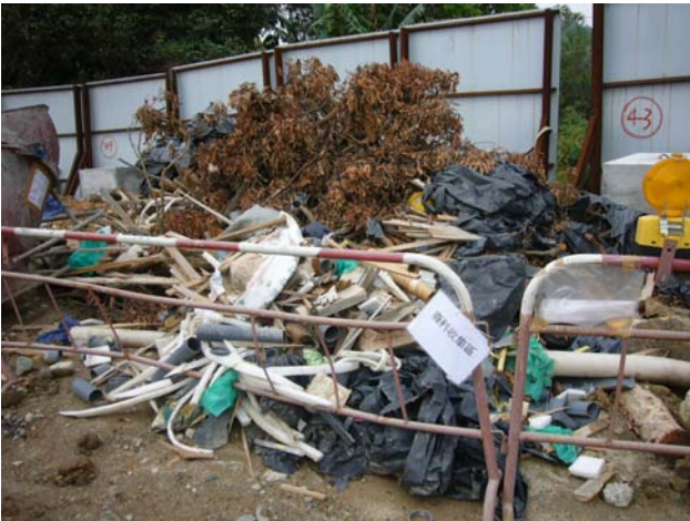
C&D waste was accumulated at the CH200, the Contractor was reminded to clean more frequency.
