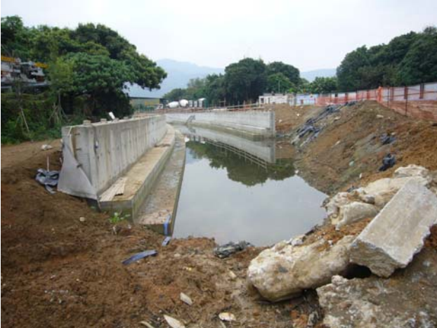
Stagnant water was accumulated at CH 200, the Contractor was reminded to clean to prevent mosquito breeding. (In progress)
