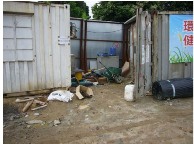
Some C&D material scattered on-site was observed at CH230, the Contractor was reminded to tight up the working area.
