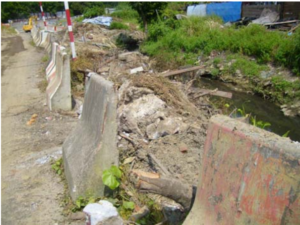
2. General and C&D waste was cumulated on site, the contractor was reminded to clean more frequency.
