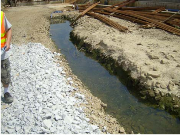
1. Stagnant waster was cumulated on site, the contractor was reminded to clean to prevent mosquito breeding
