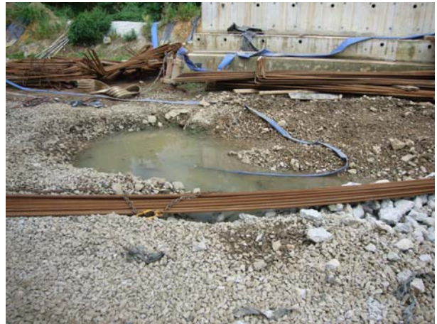
2. Stagnant water was pumping at CH-230
