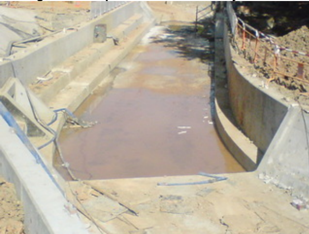
Stagnant water accumulated in the constructed channel was found at CH489. The Contractor was reminded to divert the stagnant water into the sedimentation tank prior to discharge.
