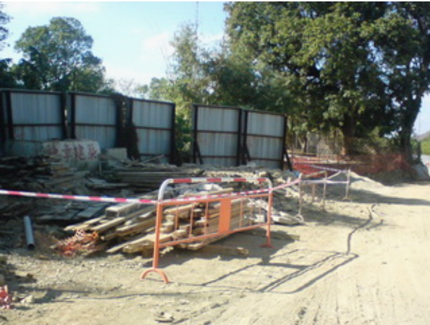
C&D waste segregation was implemented and fence off the sorting area (CH230), captioned area (CH230) had been tidy up.
