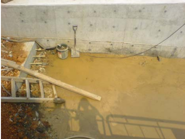
Stagnant water accumulated on-site was observed at CH130, the Contractor was reminded to clear in regular basis.
