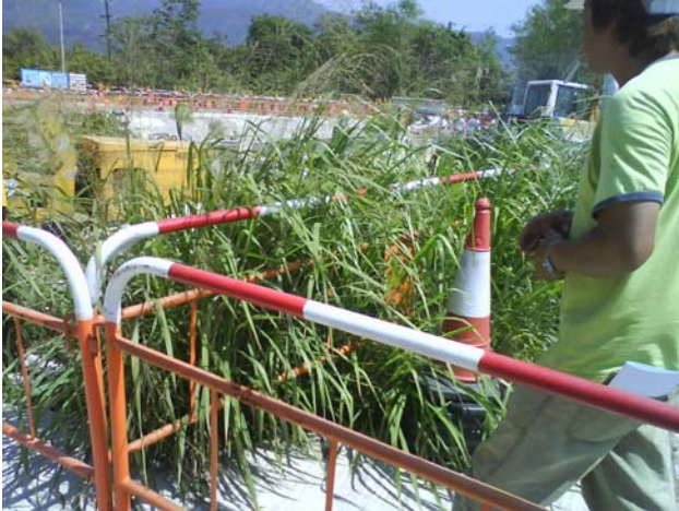
1. The weeds accumulated in Bay 1 should be removed in order to maintain the site clean and tidy.
