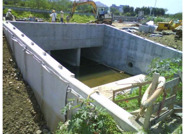
2. The stagnant water accumulated in Bay 2 should be drained away or applied larvicidal oil to prevent mosquitoes breeding.
