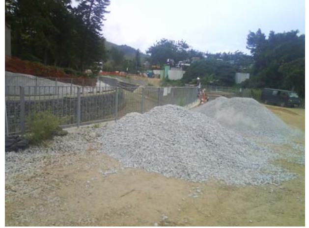
2. The gravel stockpile on the site (Ch.520) should be covered with tarpaulin sheet in order to minimize dust nuisance.
