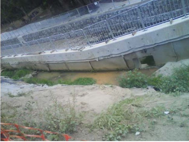
1. The stagnant water accumulated in Ch.500 should be drained away or applied larvicidal oil to prevent mosquitoes breeding.
