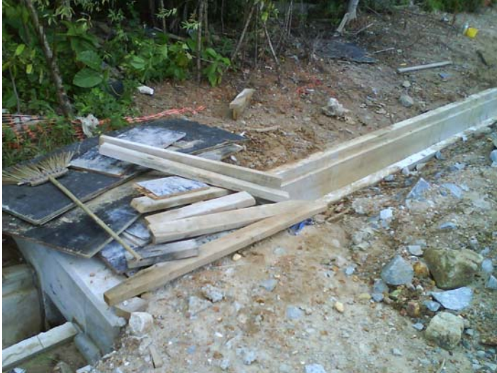
Remark 1: Used timber was observed at Ch. 200, the Contractor was reminded to improve the house keeping of the construction site.
