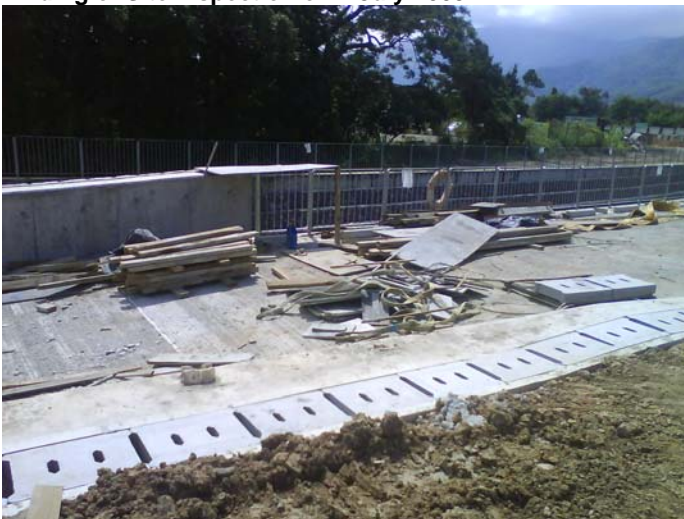
Remark 1: Scattered construction waste was observed at Ch. 300, the Contractor should improve the house keeping of the construction site.
