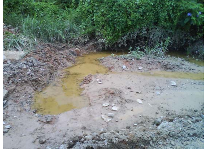
Remark 2: Stagnant water was observed at Ch. 1250, the Contractor should drain the water away to prevent mosquitoes breeding.
