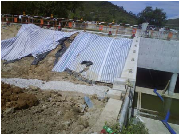
The exposed slope at the head of KT15 (Ch. 11) was found to have been covered with tarpaulin sheet.
