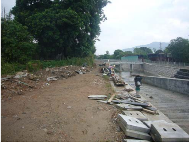
1. C&D waste was scattered on site, housingkeeping should be improved to maintain the site clean and tidy.
