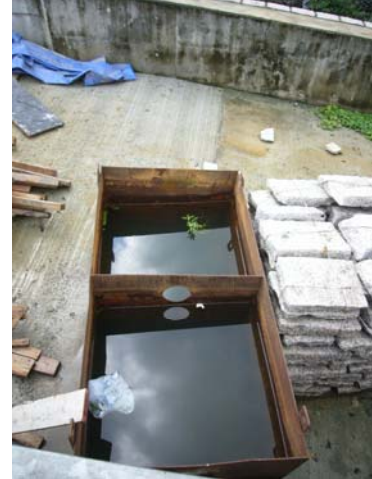
2. Stagnant water cumulated inside the unused sedimentation tank was observed at Bay 40, the Contractor was reminded to clean up to prevent mosquito breeding.
