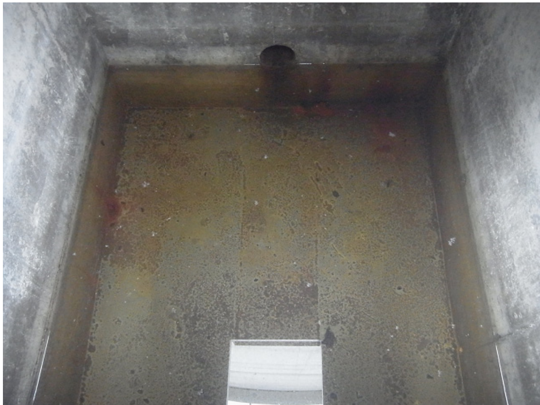
(27) Leak detection tell-tale pipe underneath the storage tank opening out to a collection chamber
