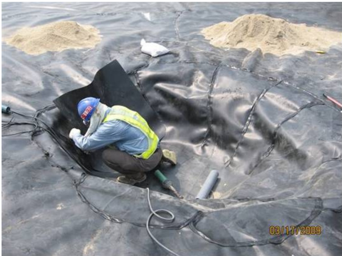
(22) Record photo shows impervious membrane laid at tank center sump with tell-tale pipe embedded for leak detection
