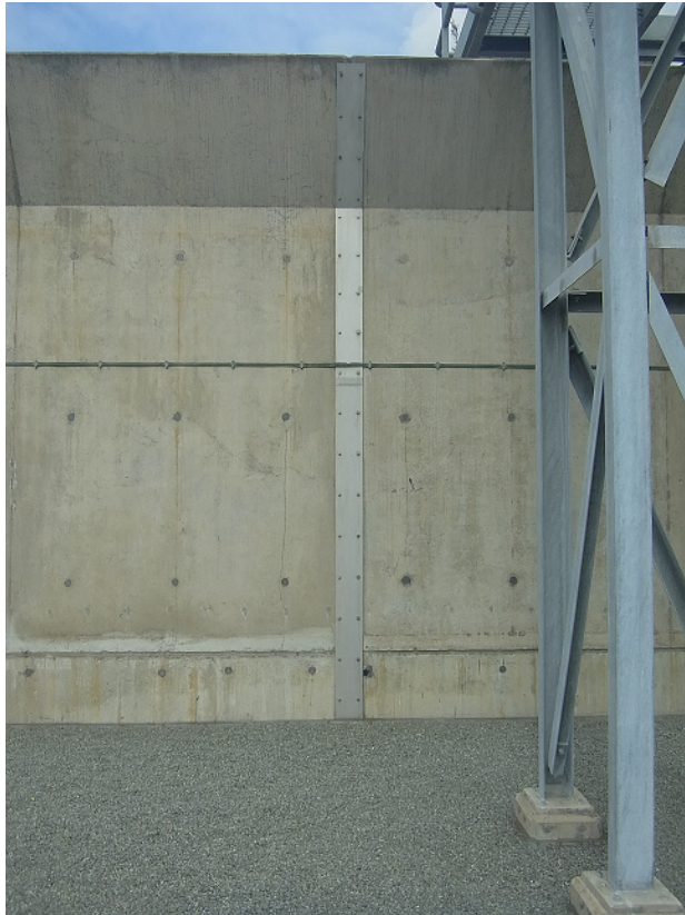
(5) Visible parts of the joints are covered by stainless steel plates on the inside at phase 1a bund
