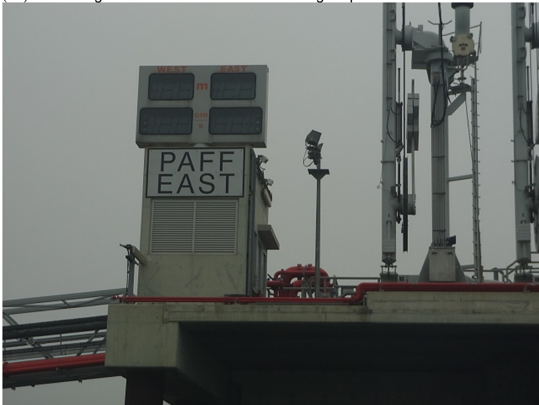
(41) Berthing aid display board installed on LP1
