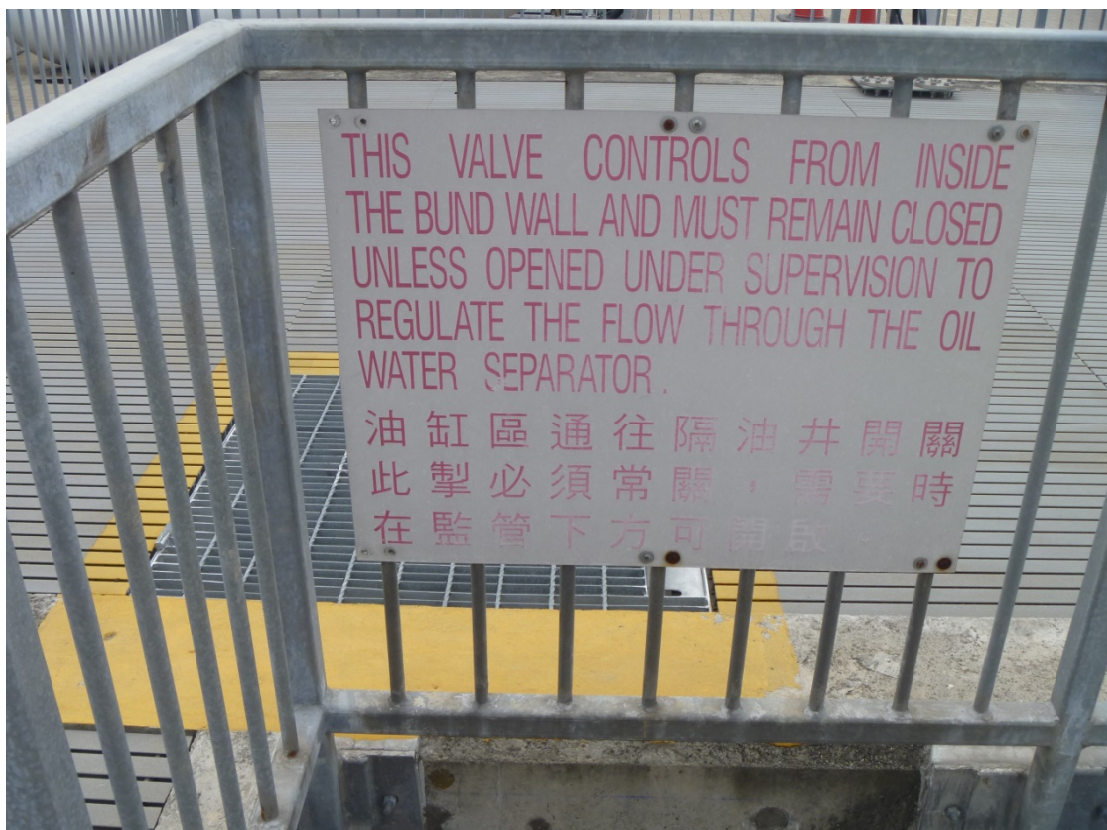
(20) Outlet valve provided for Phase 1b Interceptor with instruction sign to keep “normally closed”
