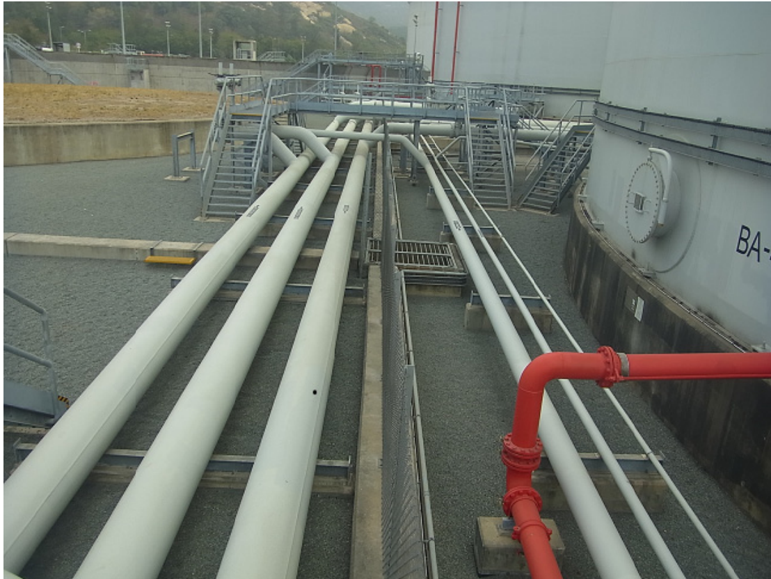
(7) Intermediate bund walls are provided in place near T-01-002
