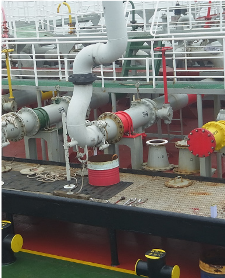
(38) Slop trays being used for coupling and de-coupling of the loading arms
