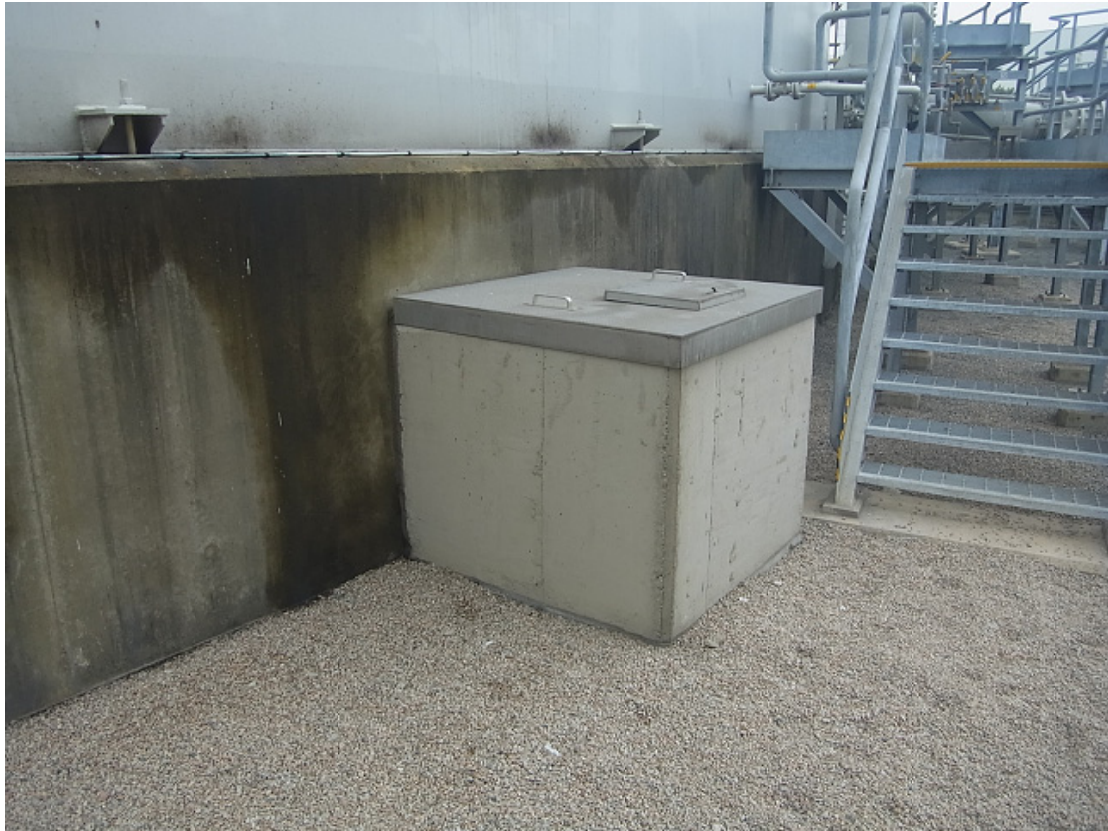
(28) Collection chamber located adjacent to tank foundation is maintained in good condition with periodic inspection
