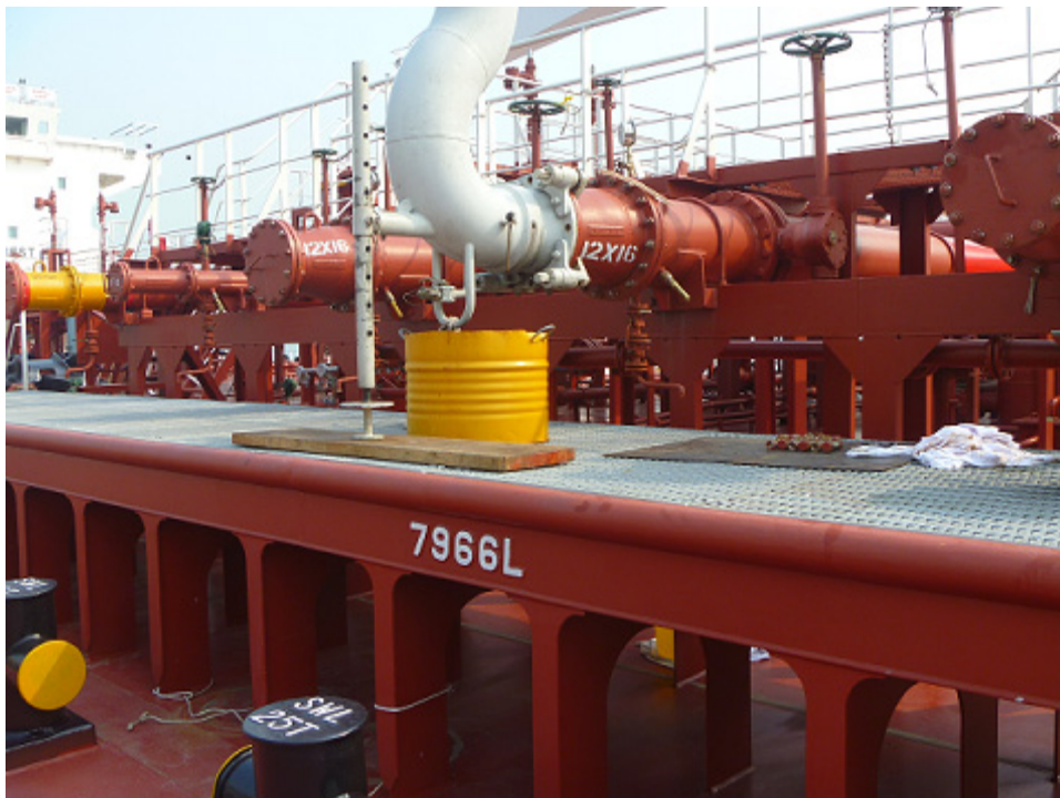
(39) Slop trays being used for coupling and de-coupling of the loading arms
