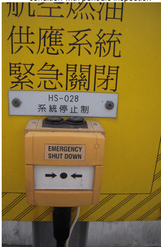
(29) ESD is maintained in good condition and being tested periodically
