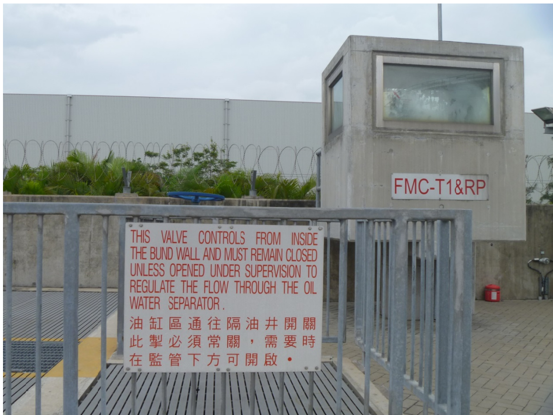
(19) Outlet valve provided for Phase 1a Interceptor with instruction sign to keep “normally closed”
