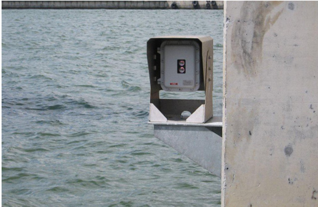
(40) Berthing aid laser box installed at Breasting Dolphin
