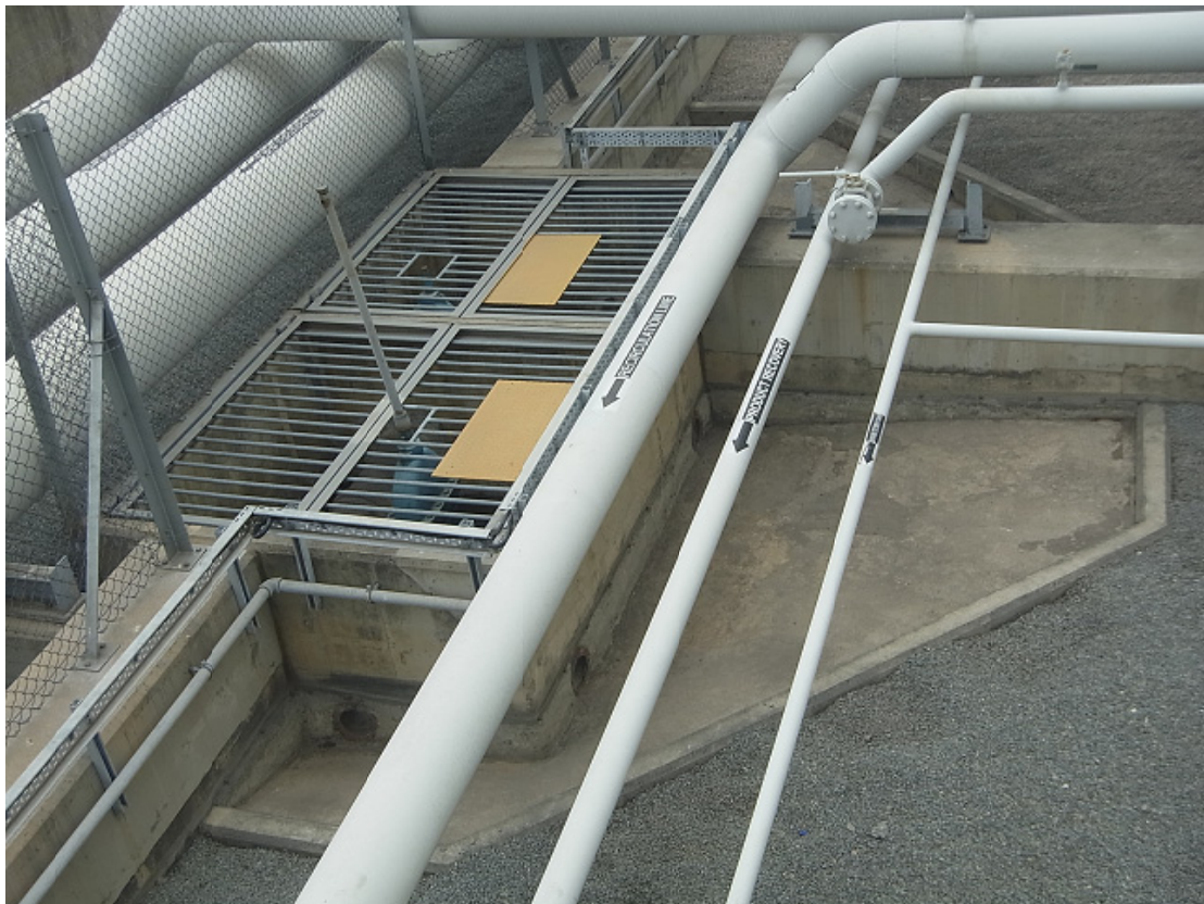
(18) Tank farm is with appropriate gradient and the drainage falls to interceptor for collection
