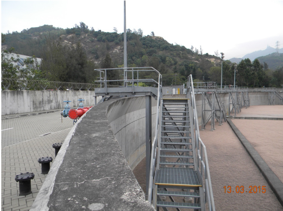
(3) Phase 1b bunded compound is partly sunken below the level of ground outside the bunds
