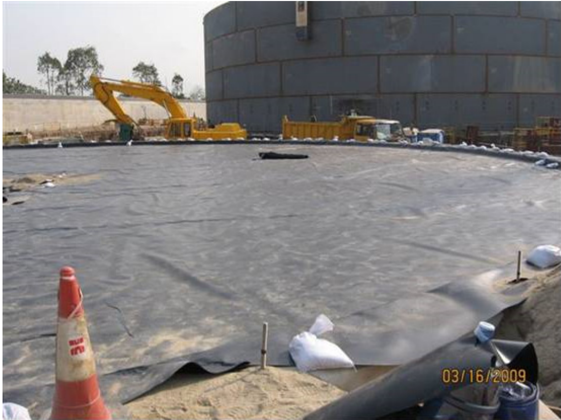
(21) Record photo shows impervious membrane being installed on top of tank foundation
