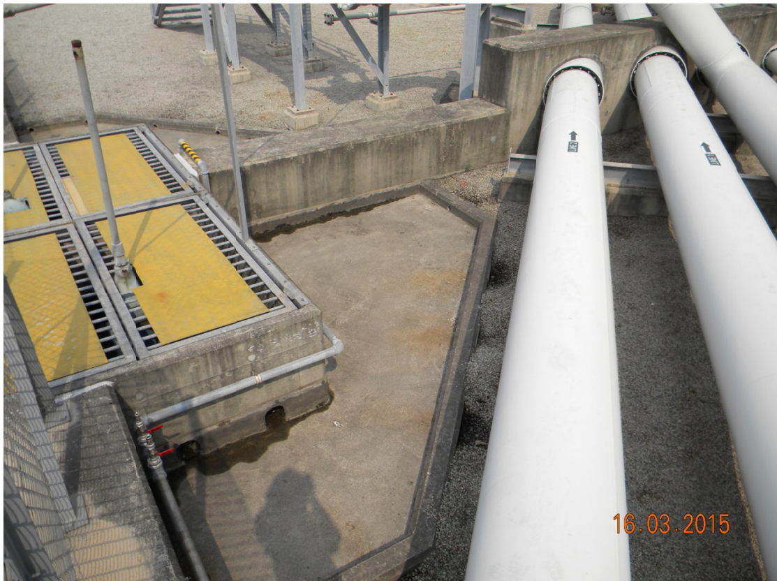
(18) Tank farm is with appropriate gradient and the drainage falls to interceptor for collection
