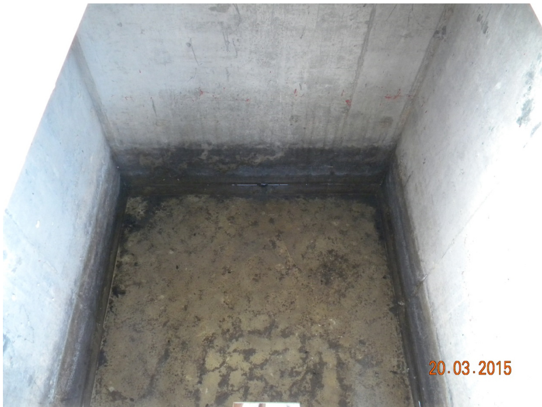
(27) Leak detection tell-tale pipe underneath the storage tank opening out to a collection chamber
