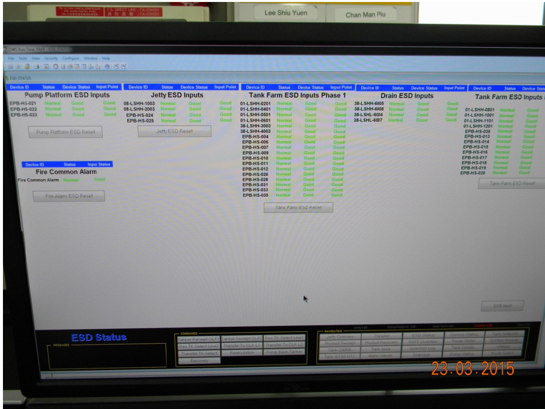
(30) The ESD regular test shown in SCADA System
