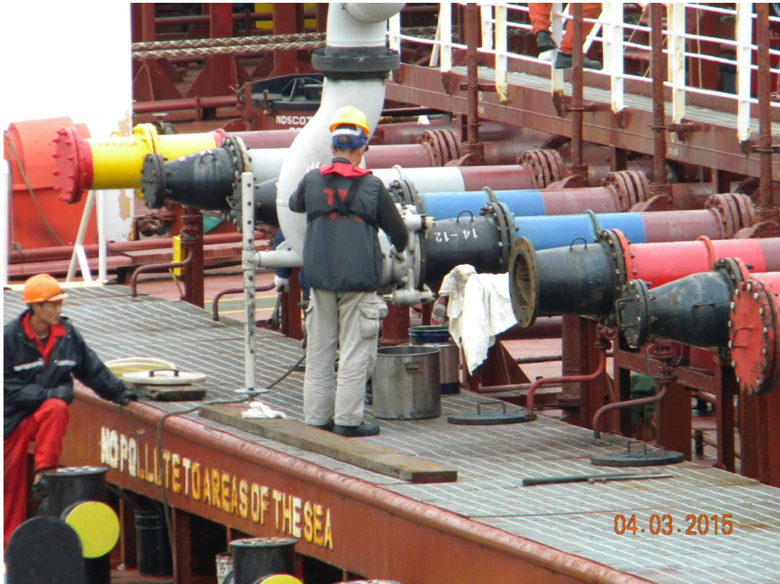
(38) Slop trays being used for coupling and de-coupling of the loading arms
