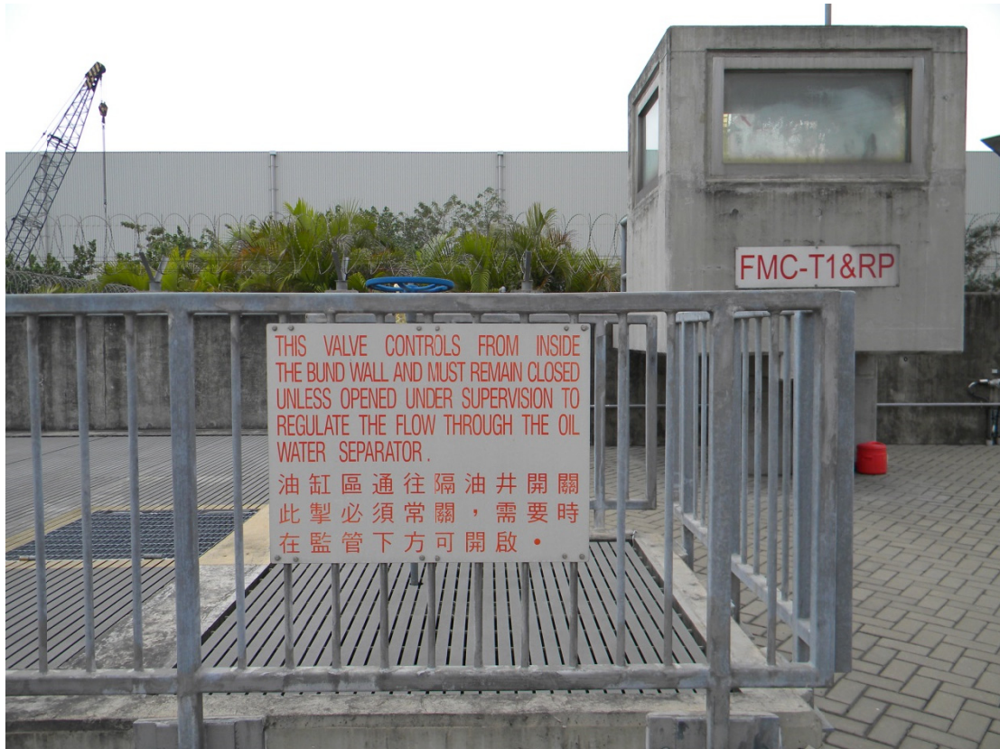
(19) Outlet valve provided for Phase 1a Interceptor with instruction sign to keep “normally closed”
