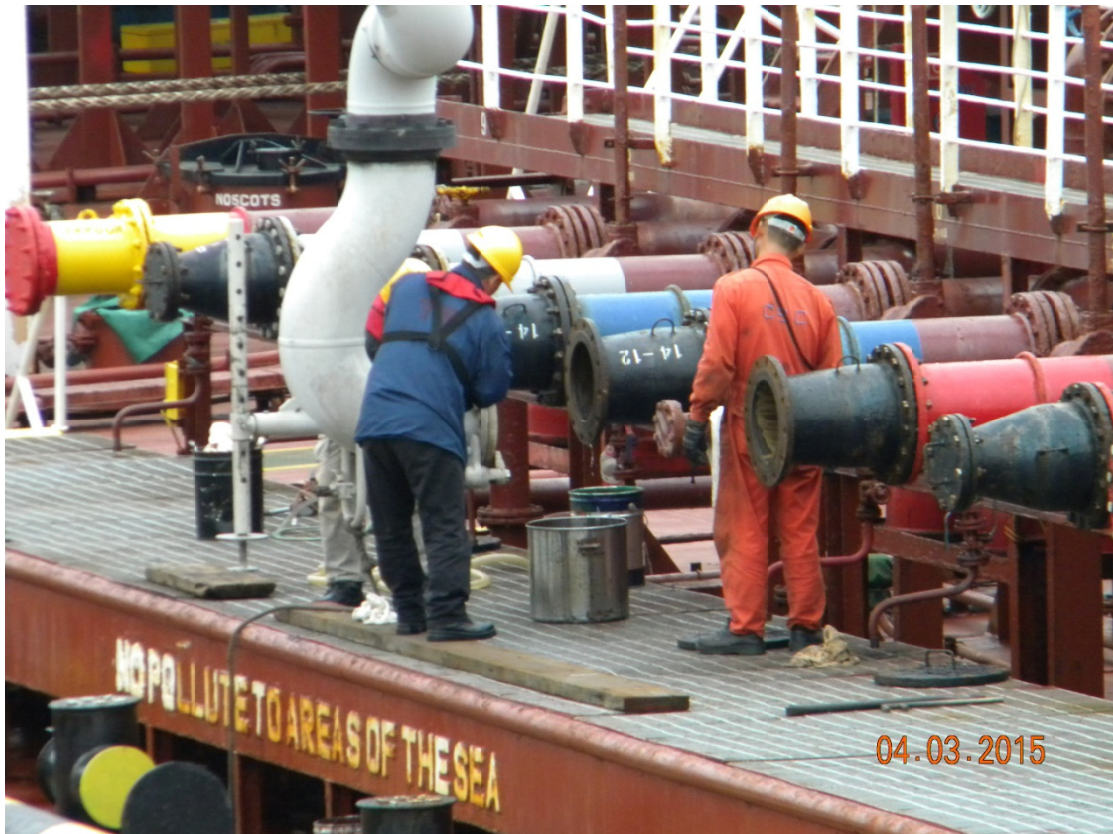
(39) Slop trays being used for coupling and de-coupling of the loading arms
