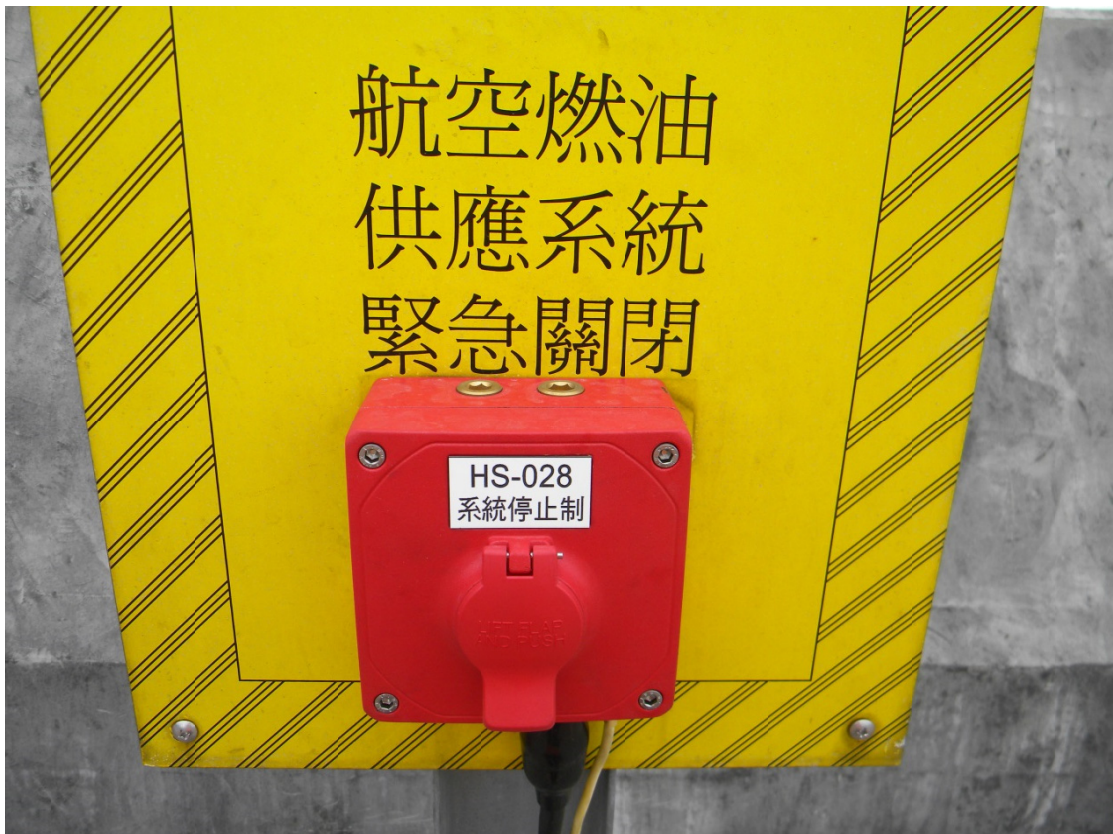
(29) ESD is maintained in good condition and being tested periodically
