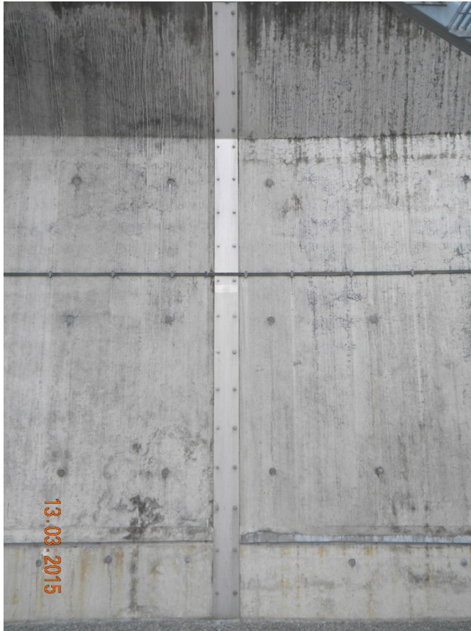
(5) Visible parts of the joints are covered by stainless steel plates on the inside at phase 1a bund
