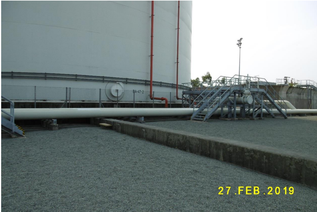
(9) Intermediate bund walls are provided in place near T-01-002
