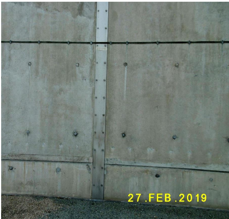
(6) Visible parts of the joints are covered by stainless steel plates on the inside at phase 1a bund
