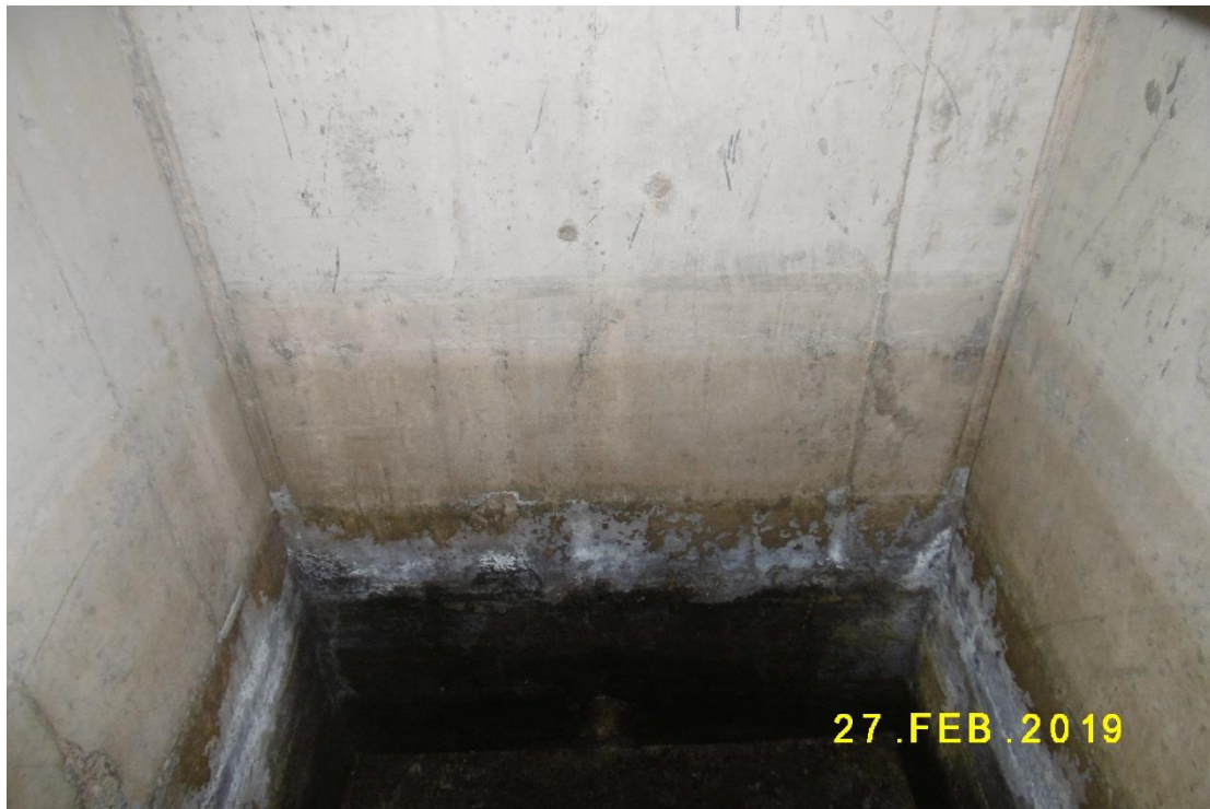
(28) Leak detection tell-tale pipe underneath the storage tank opens out to a collection chamber
