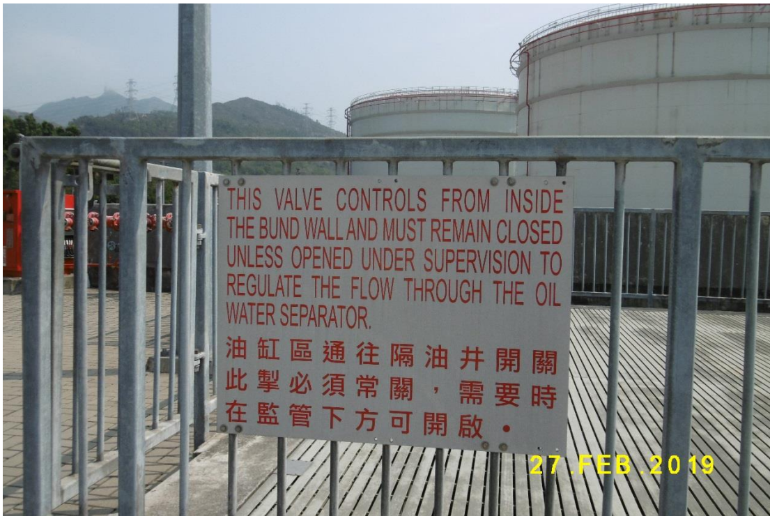
(21) Outlet valve provided for Phase 1b Interceptor with instruction sign to keep “normally closed”
