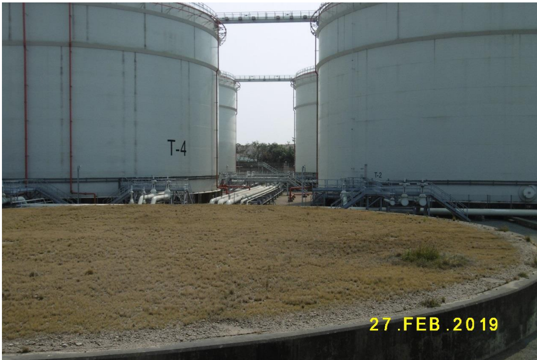
(1) Four tanks are located within bunded compound – Phase 1a
