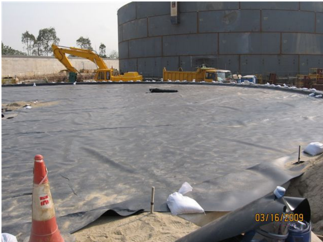
(23) Tank 16-Mar-2009 Condition of containment membrane on bottom of tank
