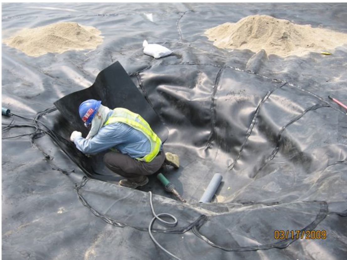
(24) Tank 17-Mar-2009 Laying membrane in center of tank T12 for sump area
