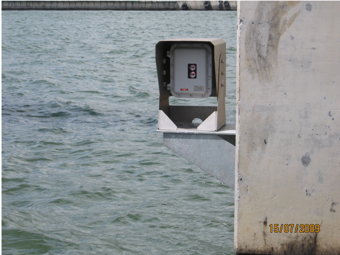
(27) BD 15-Jul-2009 Condition of laser box at BD2
