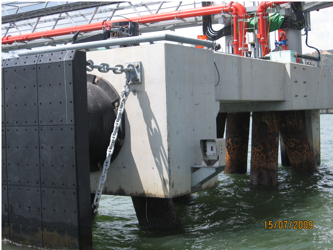
(28) BD 15-Jul-2009 Condition of laser box at BD3
