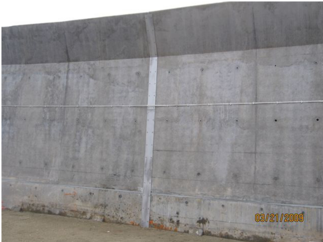
(4) Bund wall 21-Mar-2009 Condition of fire resistance steel plate installation on wall joint
