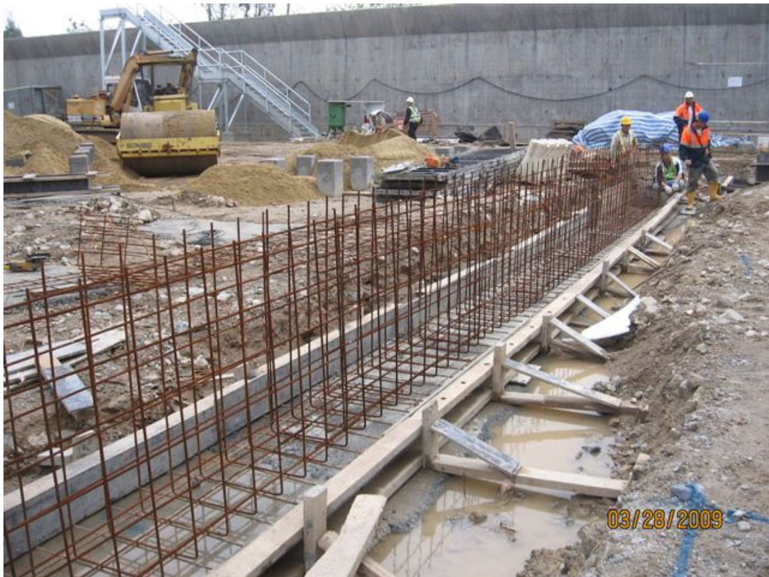
(8) Bund wall 28-Mar-2009 Steel mesh condition for internal bund wall between T6 & T5
