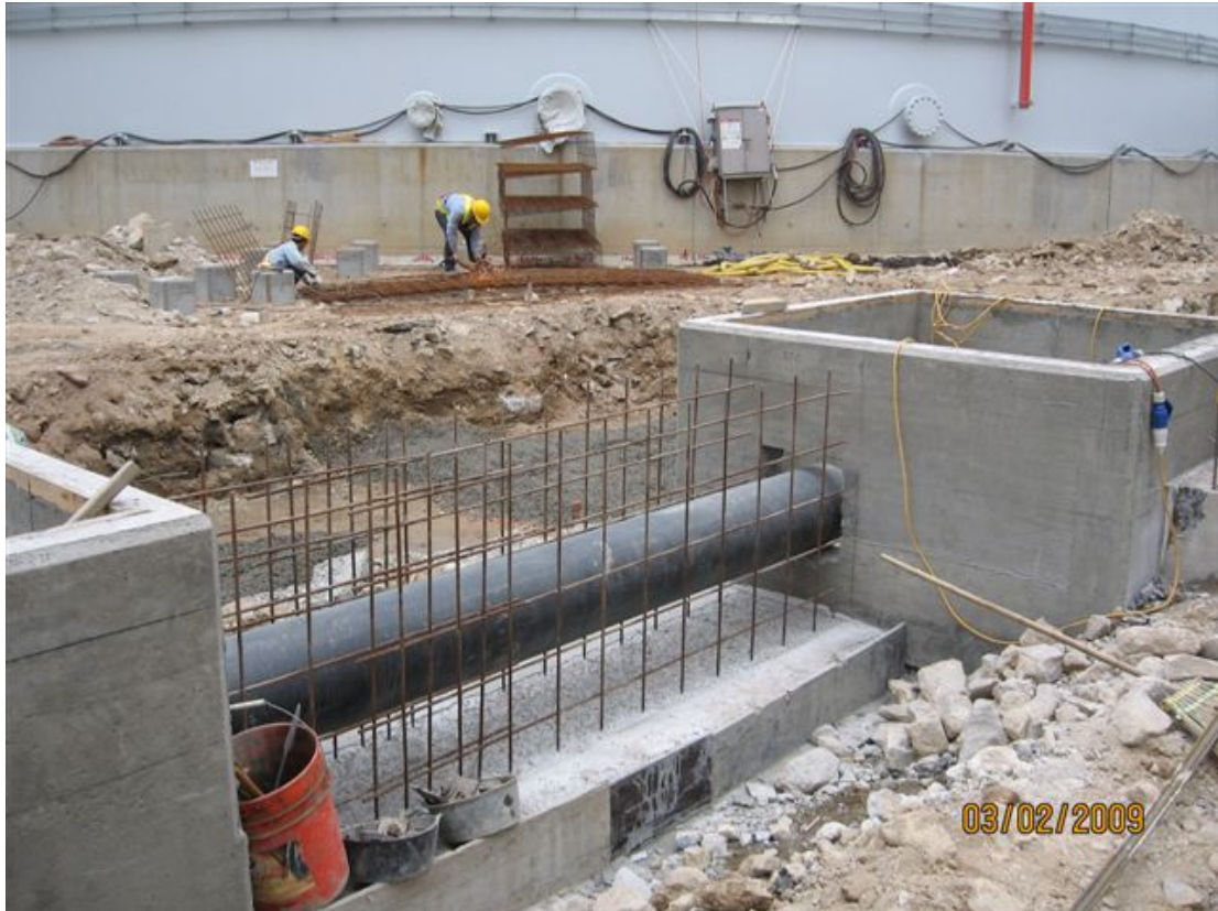
(9) Drainage 2-Mar-2009 Condition of drainage pipe & catch pit connect to internal bund wall
