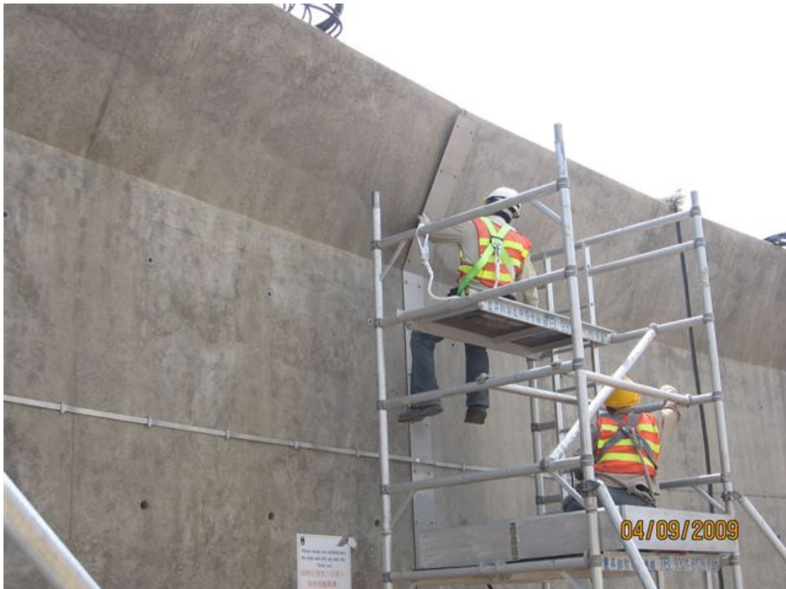
(6) Bund wall 9-Apr-2009 Erecting steel fire resistance plate at movement joint of wall
