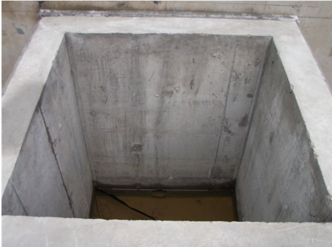
(21) Leak detection pipe underneath the storage tank opening out to a containment 15-Jul-2009
