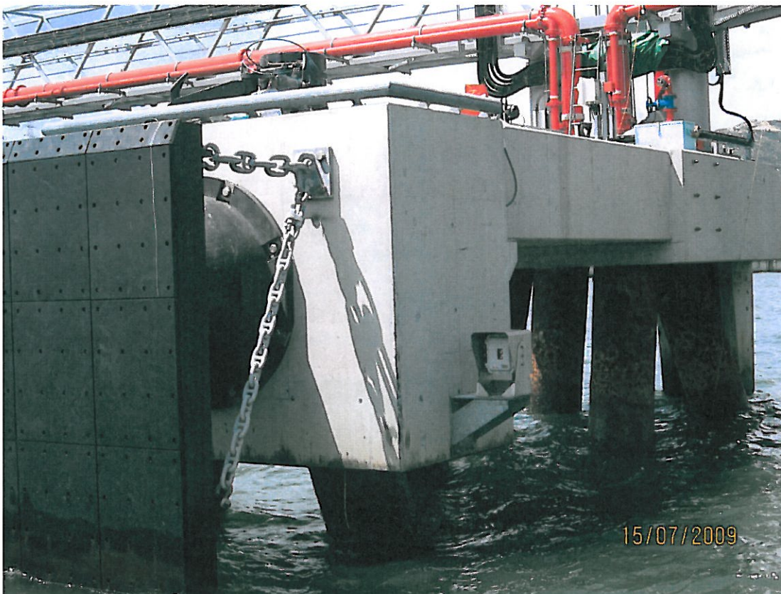
(28) BD 15-Jul-2009 Condition of laser box at BD3
