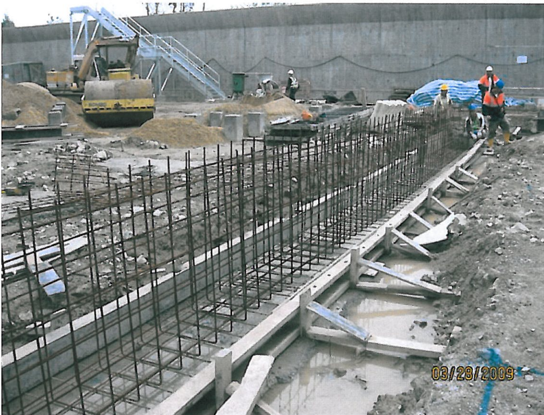
(8) Bund wall 28-Mar-2009 Steel mesh condition for internal bund wall between T6 & T5
