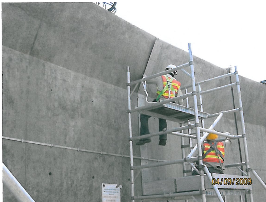
(6) Bund wall 9-Apr-2009 Erecting steel fire resistance plate at movement joint of wall
