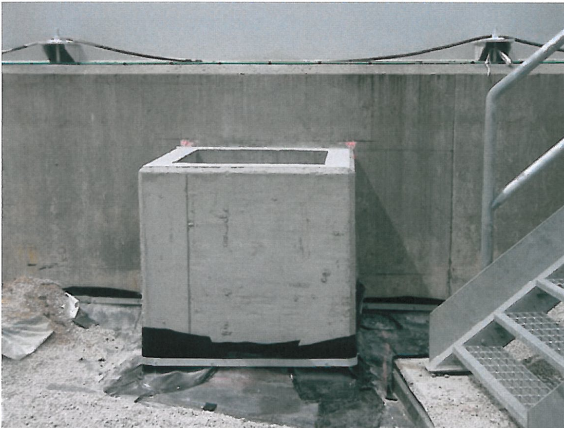
(20) Containment for leak detection of the bottom of storage tank 15-Jul-2009
