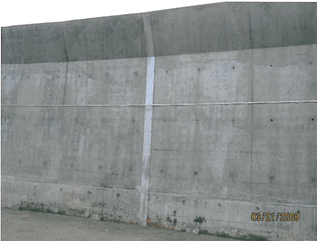
(4) Bund wall 21-Mar-2009 Condition of fire resistance steel plate installation on wall joint
