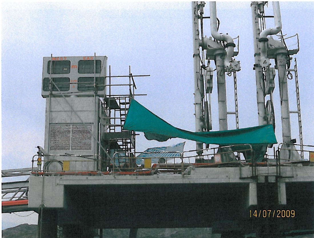
(29) LP2 14-Jul-2009 General view for display board on LP1
