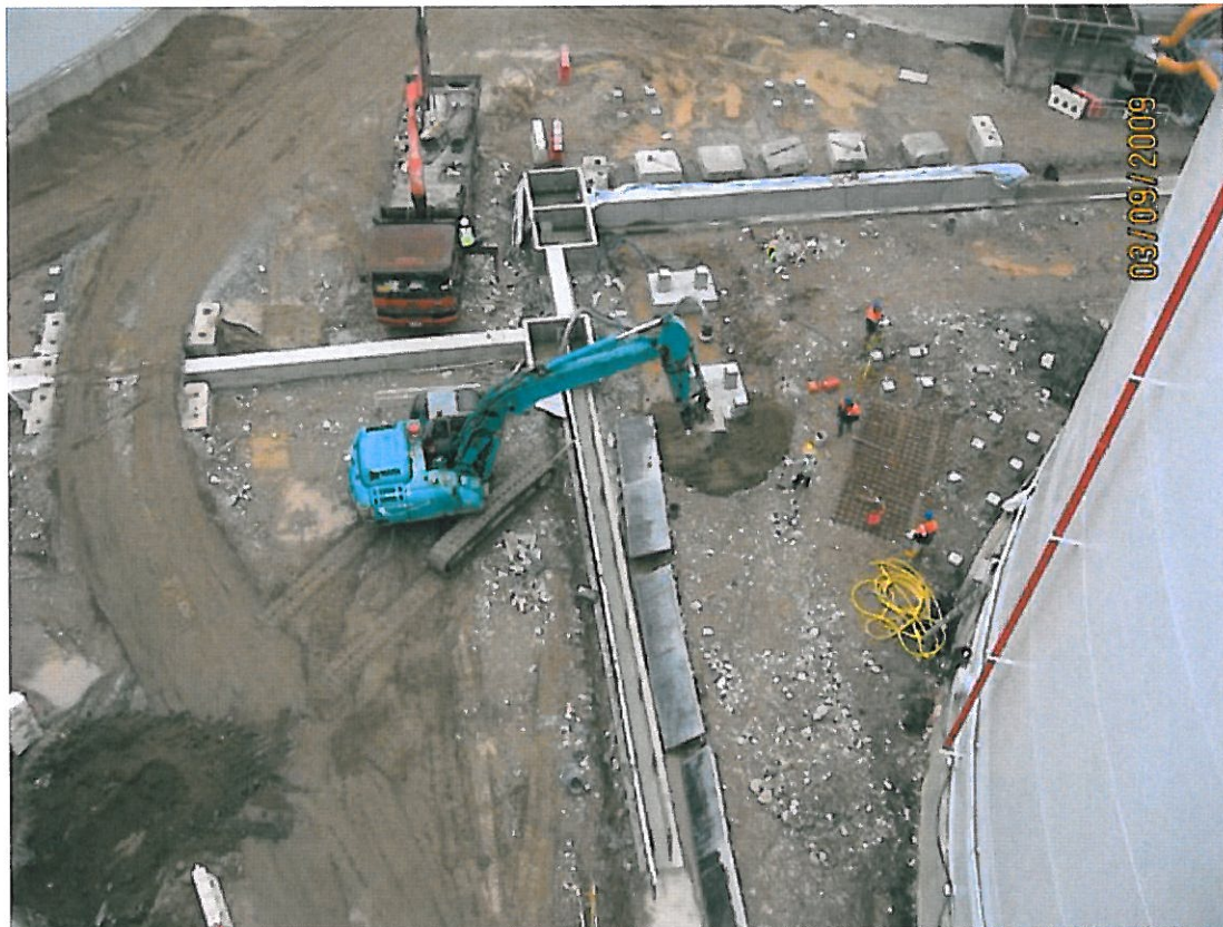
(2) Bund area 9-Mar-2009 General view for internal bund wall between T2 & T5
