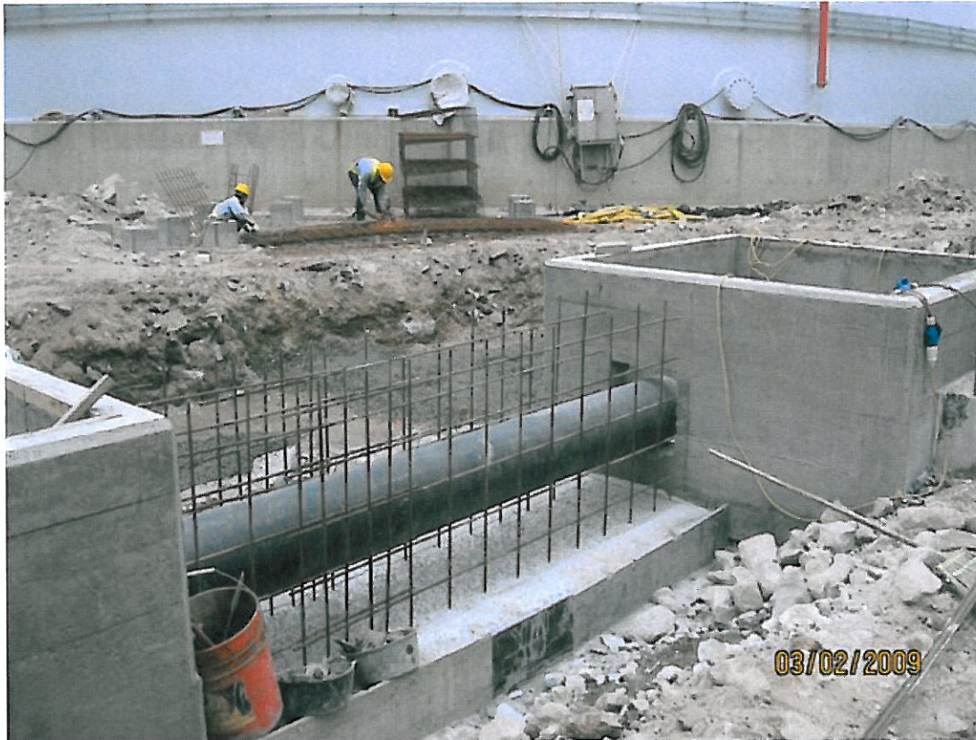
(9) Drainage 2-Mar-2009 Condition of drainage pipe & catch pit connect to internal bund wall
