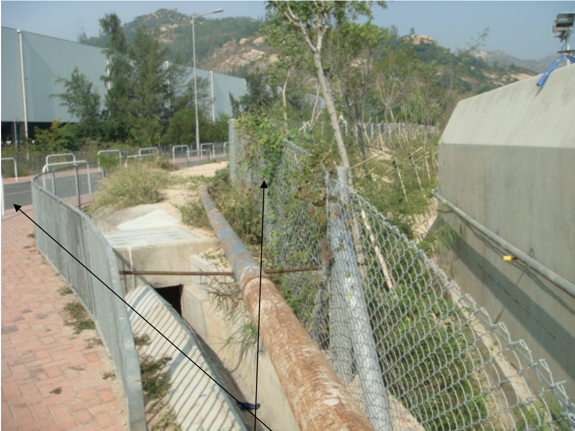
View of section Y-Y. Note that the height of the road is lower than the height of the landscape bund.
