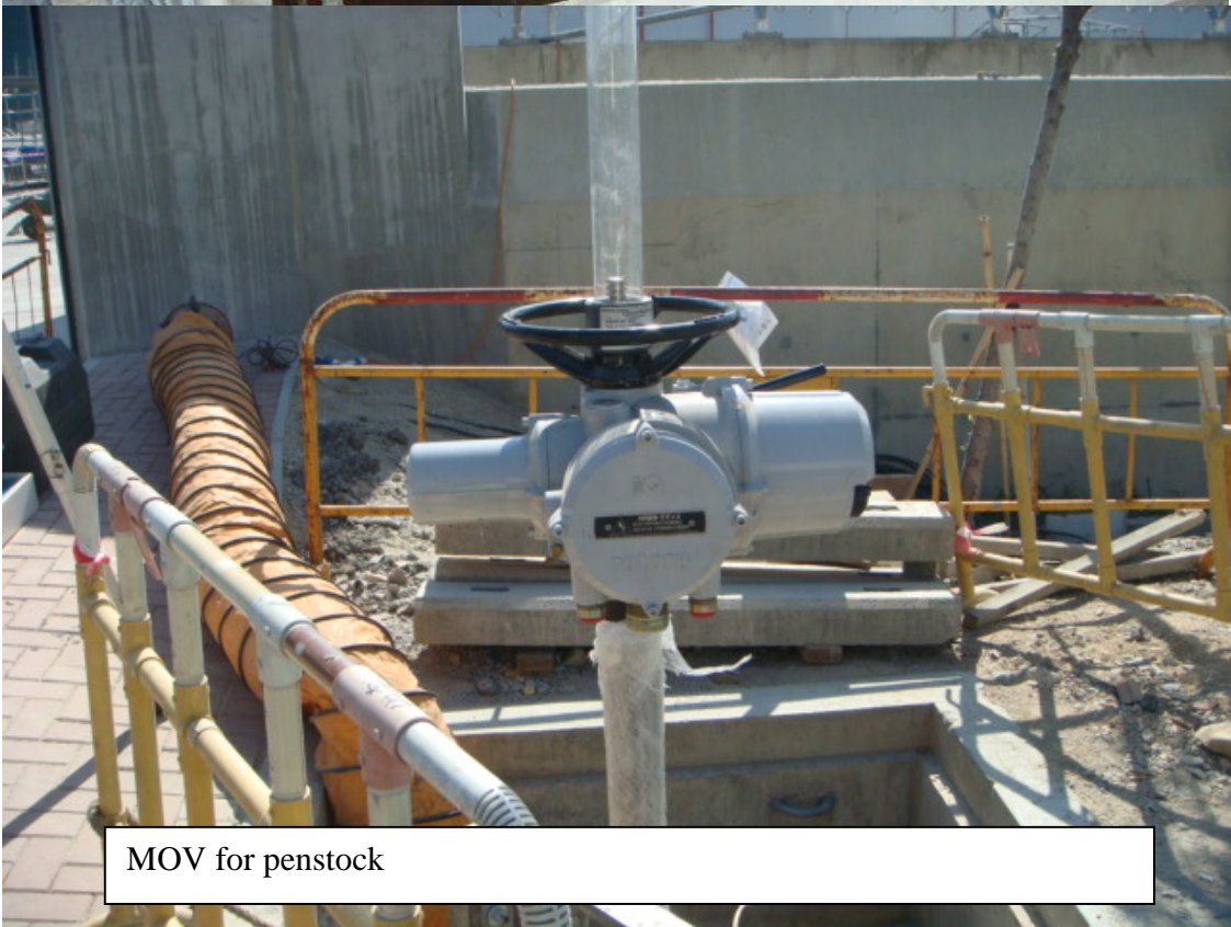
Penstock at final stormwater manhole
