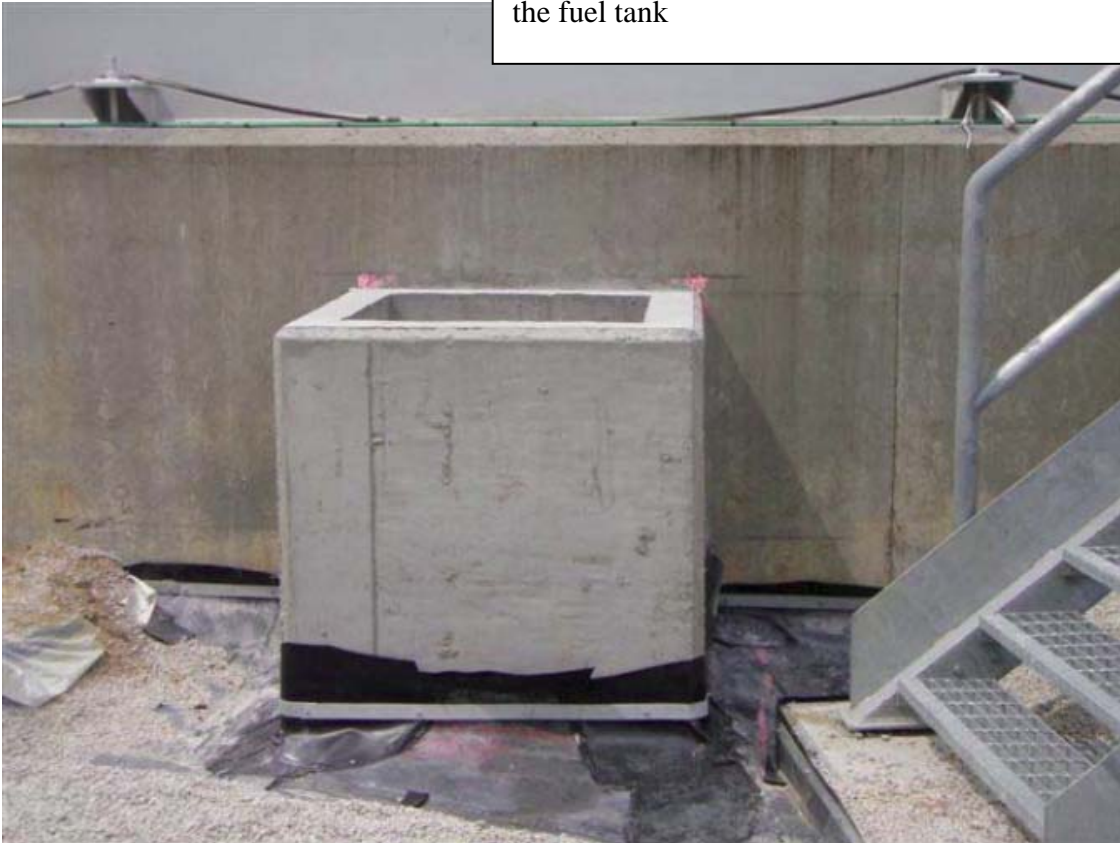
Receipt chamber for leak detection pipe outlet at bottom of fuel tank
