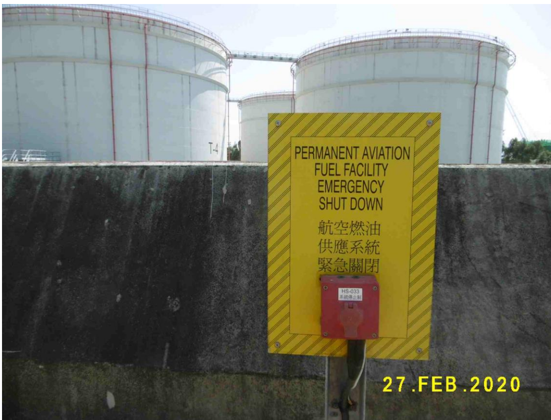
(30) ESD device is maintained in good condition and being tested periodically
