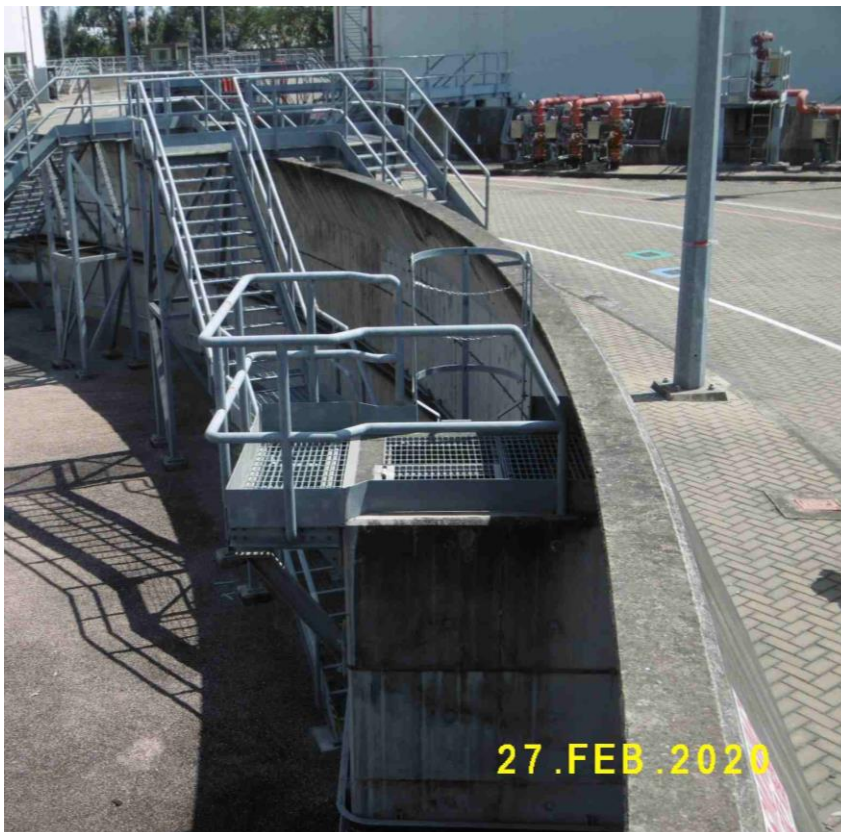
(4) Phase 1b bunded compound is lower than the ground level outside the bunds
