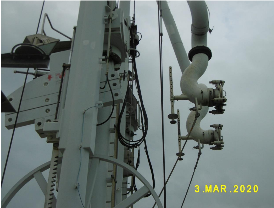
(39) Slop collection utilities are used for coupling and de-coupling of the loading arms
