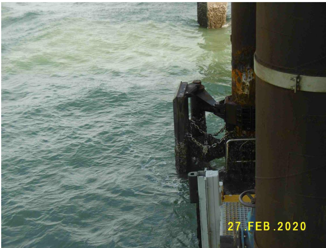
(38) Fenders are installed at shore side of the jetty
