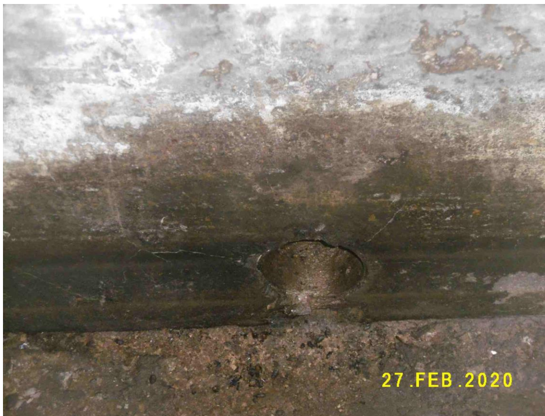
(28) Leak detection tell-tale pipe underneath the storage tank opens out to a collection chamber
