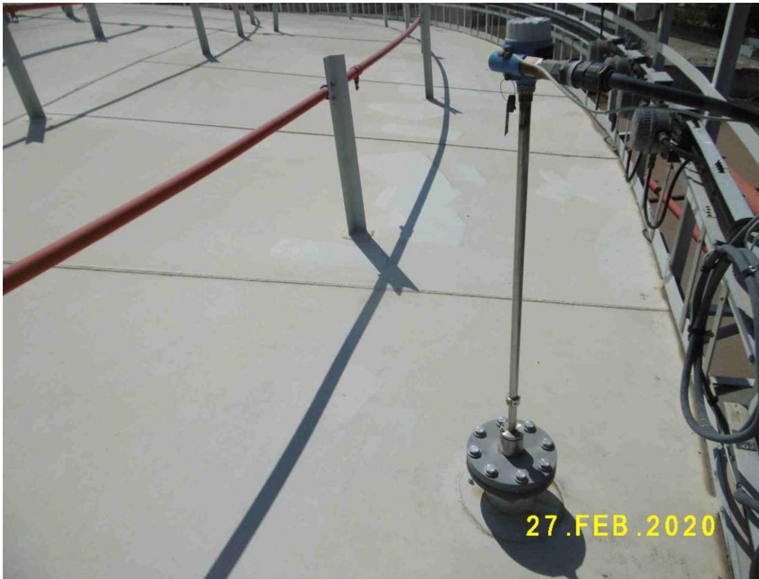
(25) Regular inspection performed on overfilling monitoring device (High-High Level Alarm)
