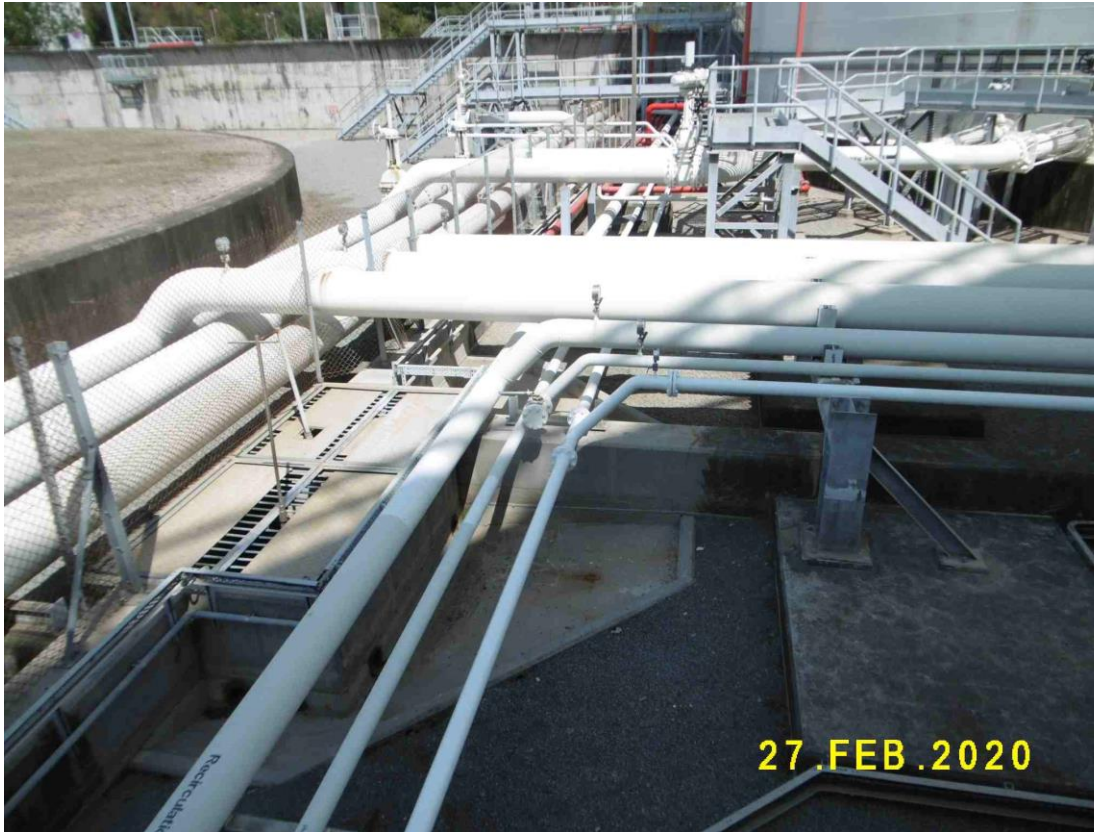
(19) Tank farm is with appropriate gradient and the drainage falls to interceptor for collection
