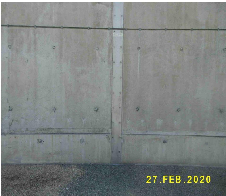
(6) Visible parts of the joints are covered by stainless steel plates on the inside at phase 1a bund
