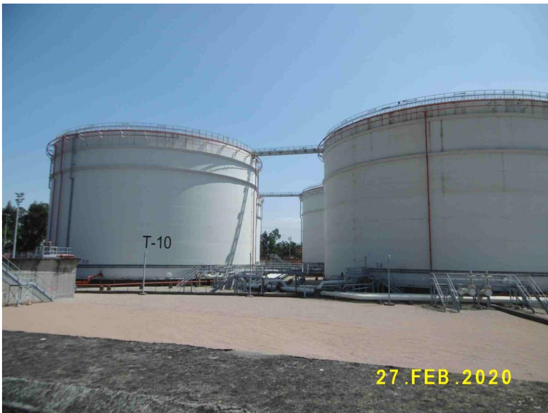
(2) Four tanks are located within bunded compound – Phase 1b
