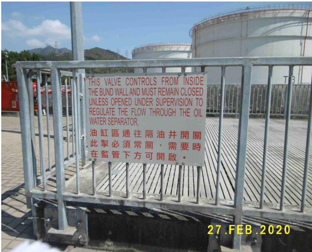
(21) Outlet valve provided for Phase 1b Interceptor with instruction sign to keep “normally closed”
