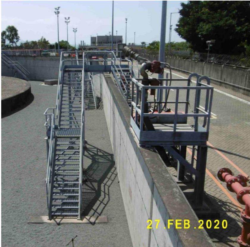
(3) Phase 1a bunded compound is lower than the ground level outside the bunds
