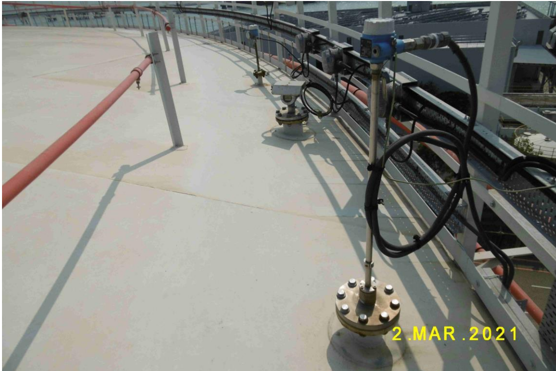
(25) Regular inspection performed on overfilling monitoring device (High-High Level Alarm)
