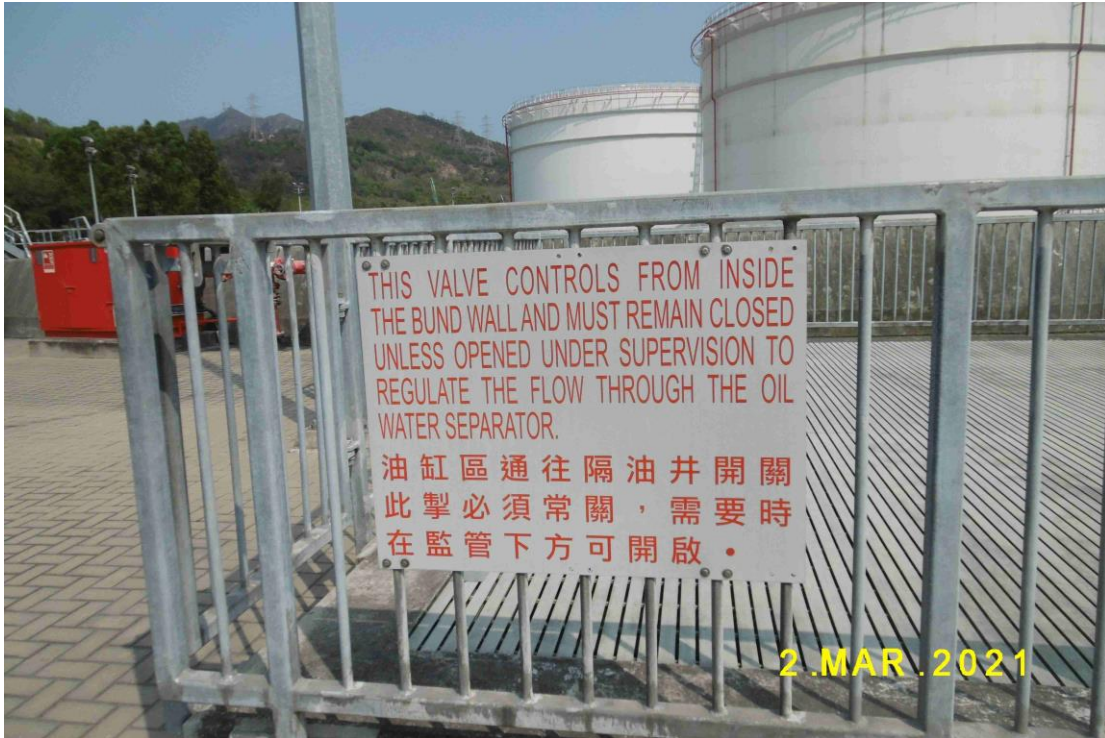
(21) Outlet valve provided for Phase 1b Interceptor with instruction sign to keep “normally closed”
