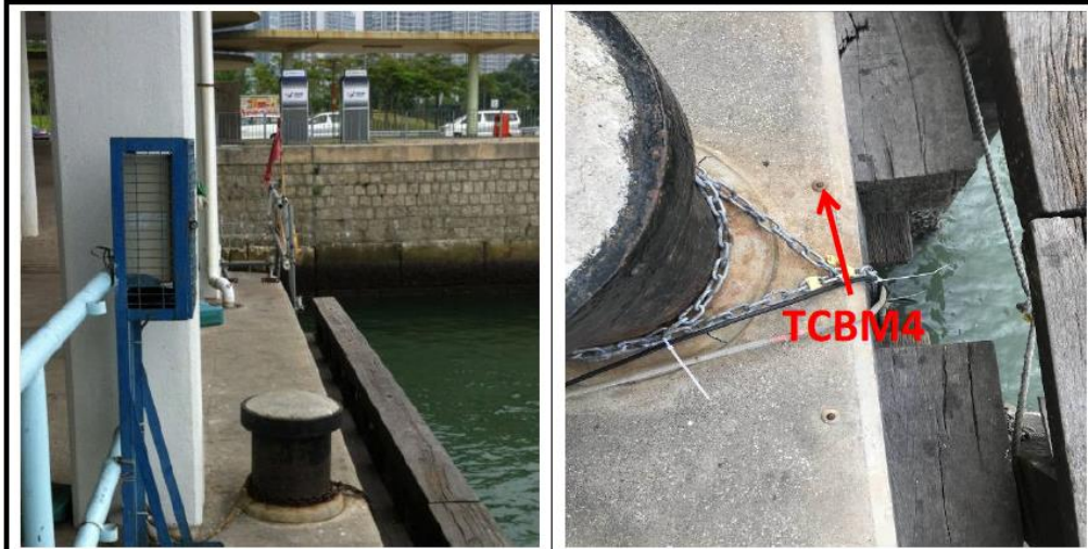
Plate 5: Project tide gauge installed at the shore of Tung Chung Development Pier
