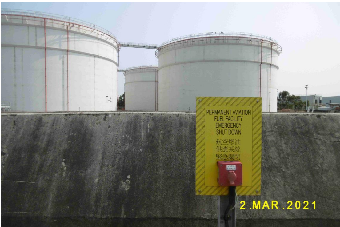
(30) ESD device is maintained in good condition and being tested periodically
