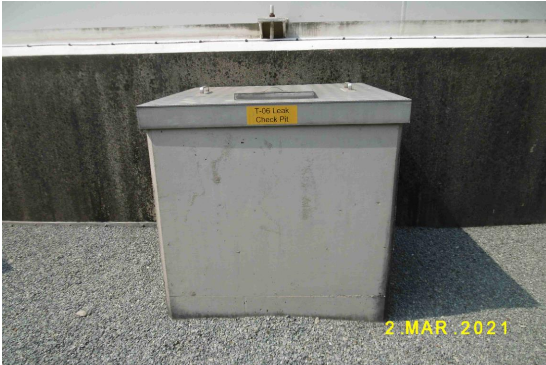
(29) Collection chamber located adjacent to tank foundation is maintained in good condition with periodic inspection
