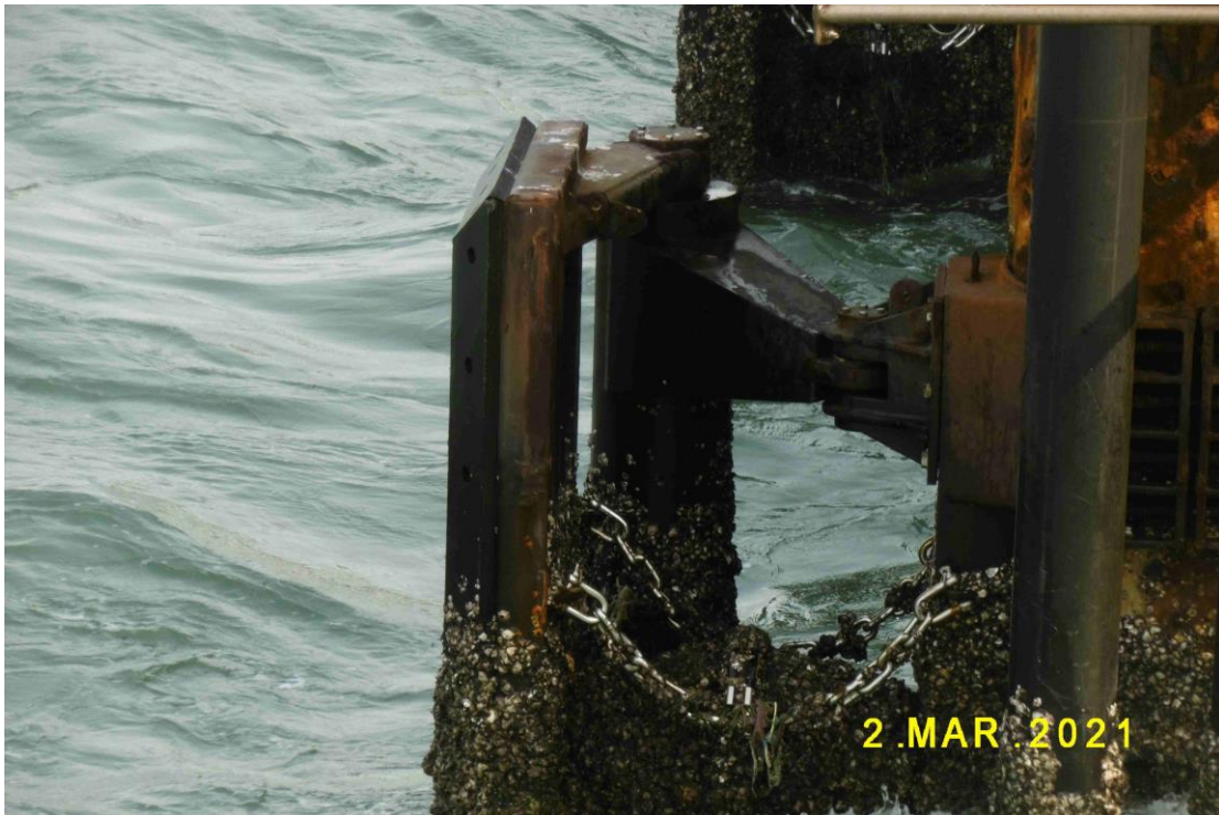
(38) Fenders are installed at shore side of the jetty
