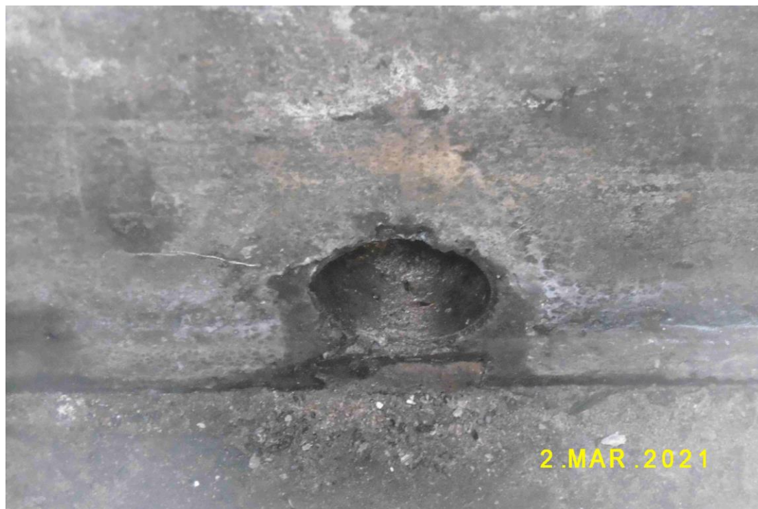
(28) Leak detection tell-tale pipe underneath the storage tank opens out to a collection chamber
