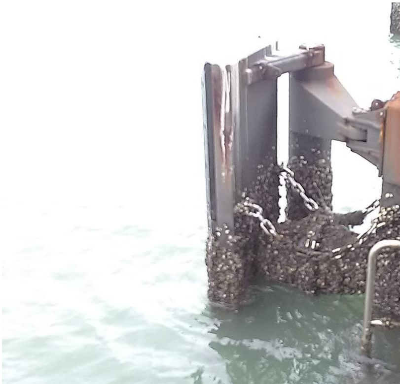
(38) Fenders are installed at shore side of the jetty
