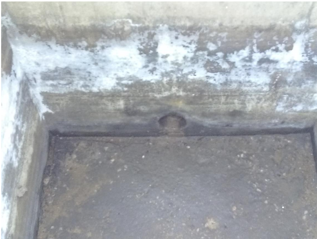
(28) Leak detection tell-tale pipe underneath the storage tank opens out to a collection chamber
