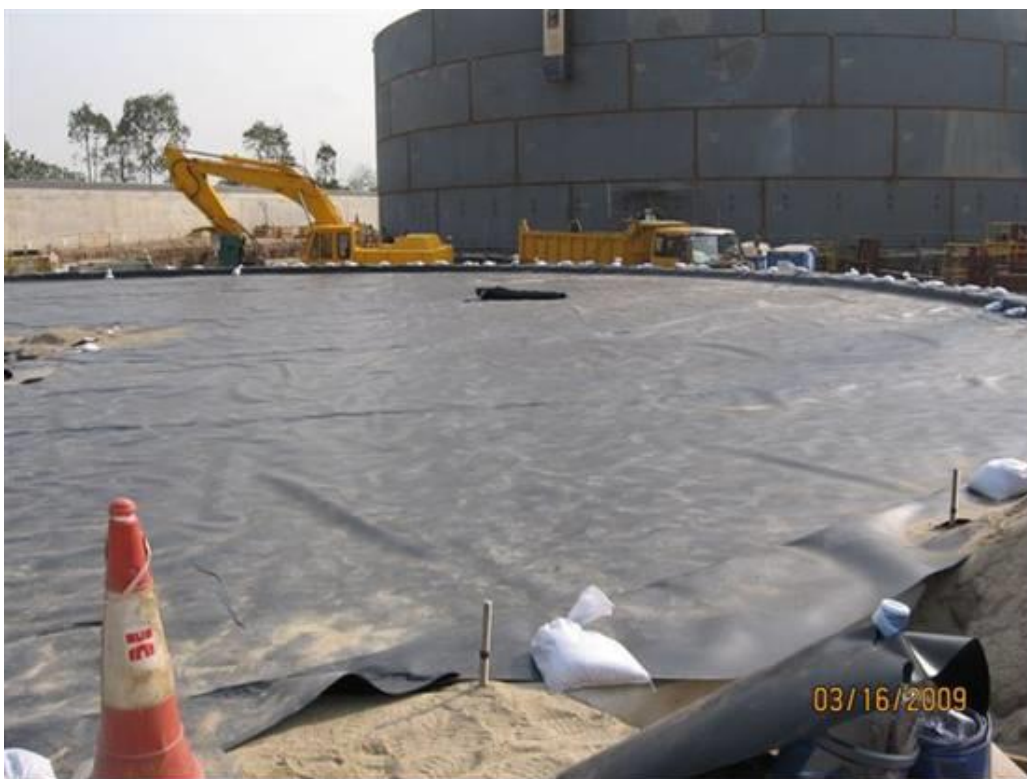
(22) Record photo shows impervious membrane being installed on top of tank foundation
