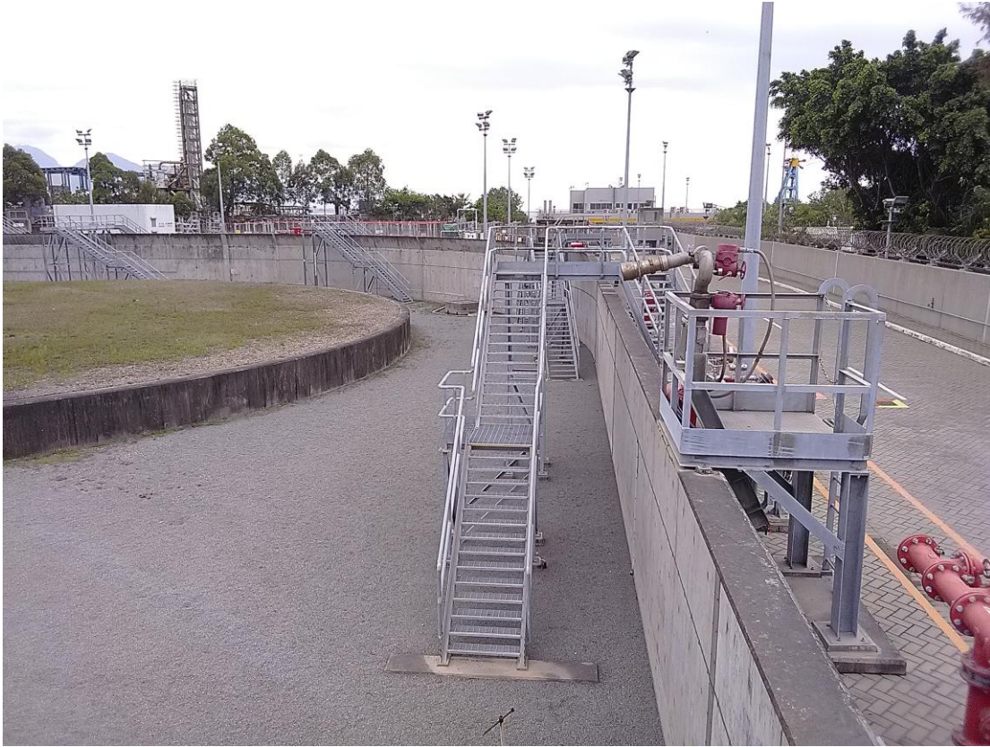
(3) Phase 1a bunded compound is lower than the ground level outside the bunds
