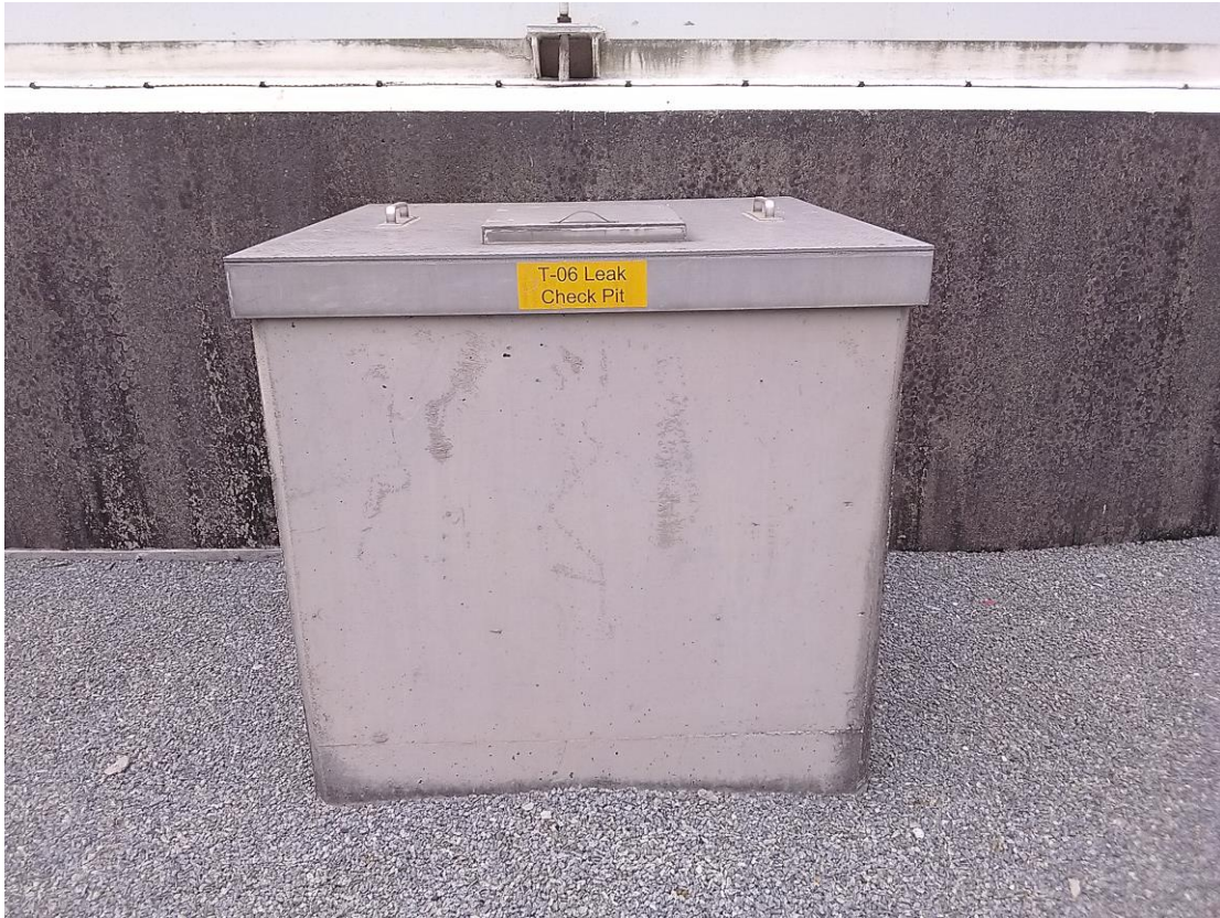
(29) Collection chamber located adjacent to tank foundation is maintained in good condition with periodic inspection
