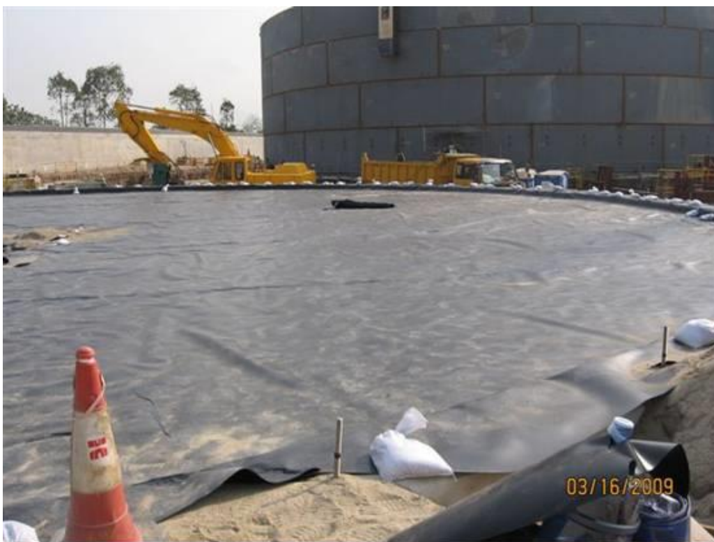
(22) Record photo shows impervious membrane being installed on top of tank foundation
