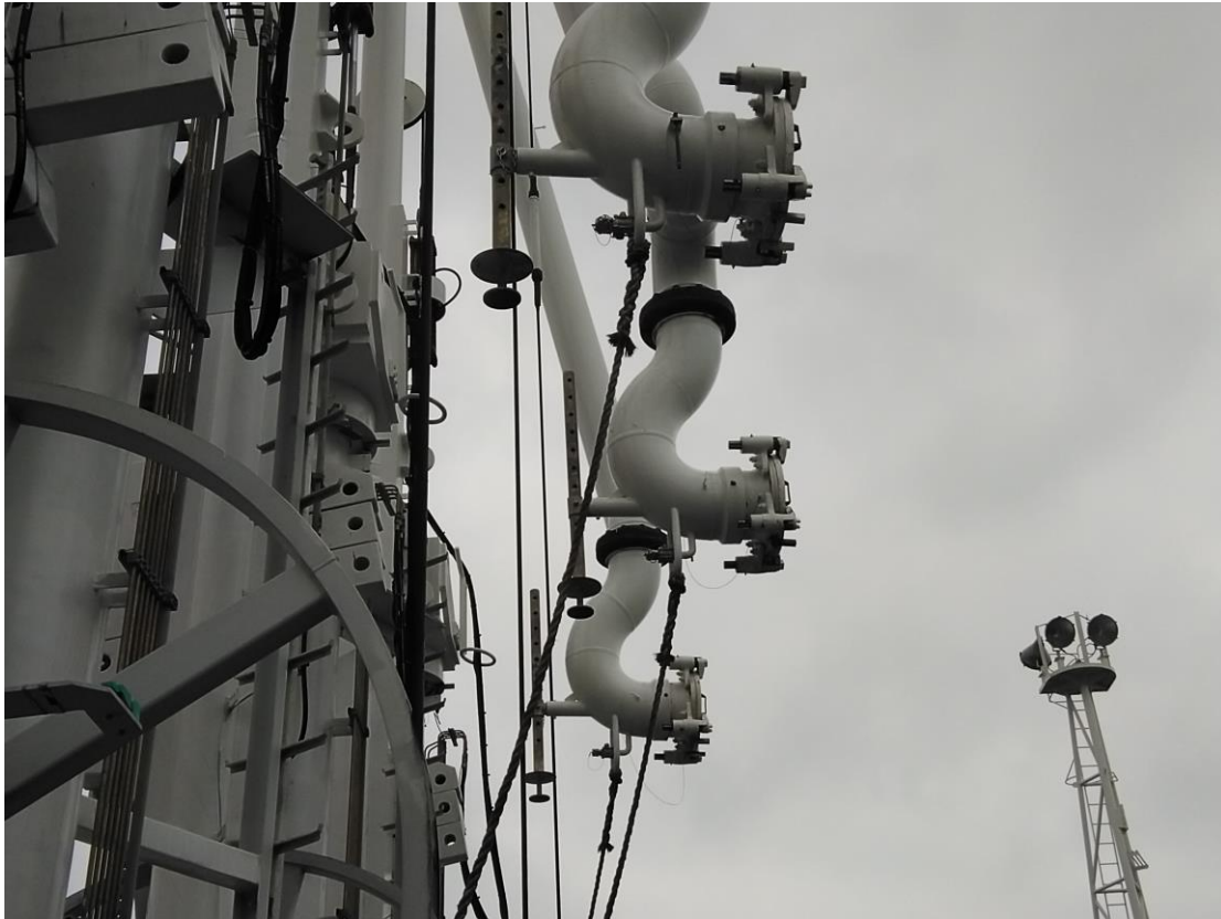
(39) Slop collection utilities are used for coupling and de-coupling of the loading arms
