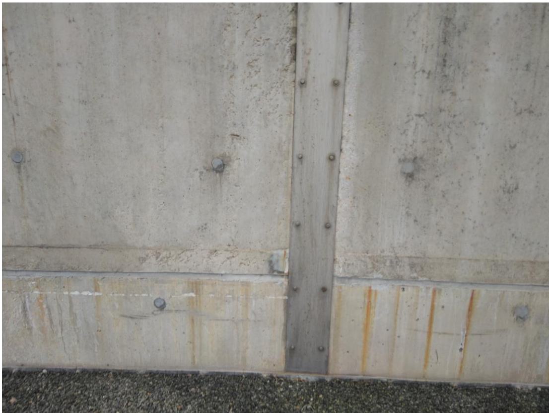
(6) Visible parts of the joints are covered by stainless steel plates on the inside at phase 1a bund
