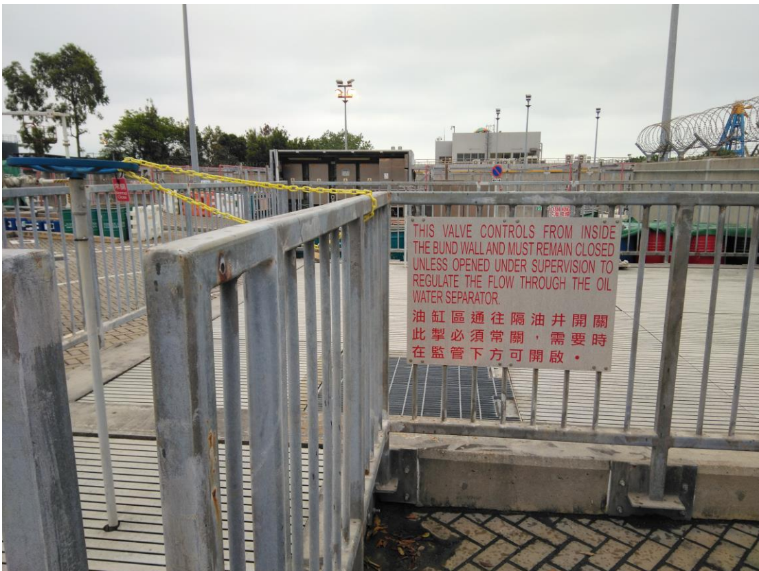
(20) Outlet valve provided for Phase 1a Interceptor with instruction sign to keep “normally closed”
