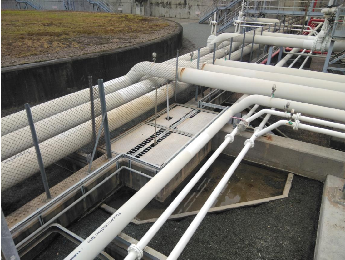
(19) Tank farm is with appropriate gradient and the drainage falls to interceptor for collection
