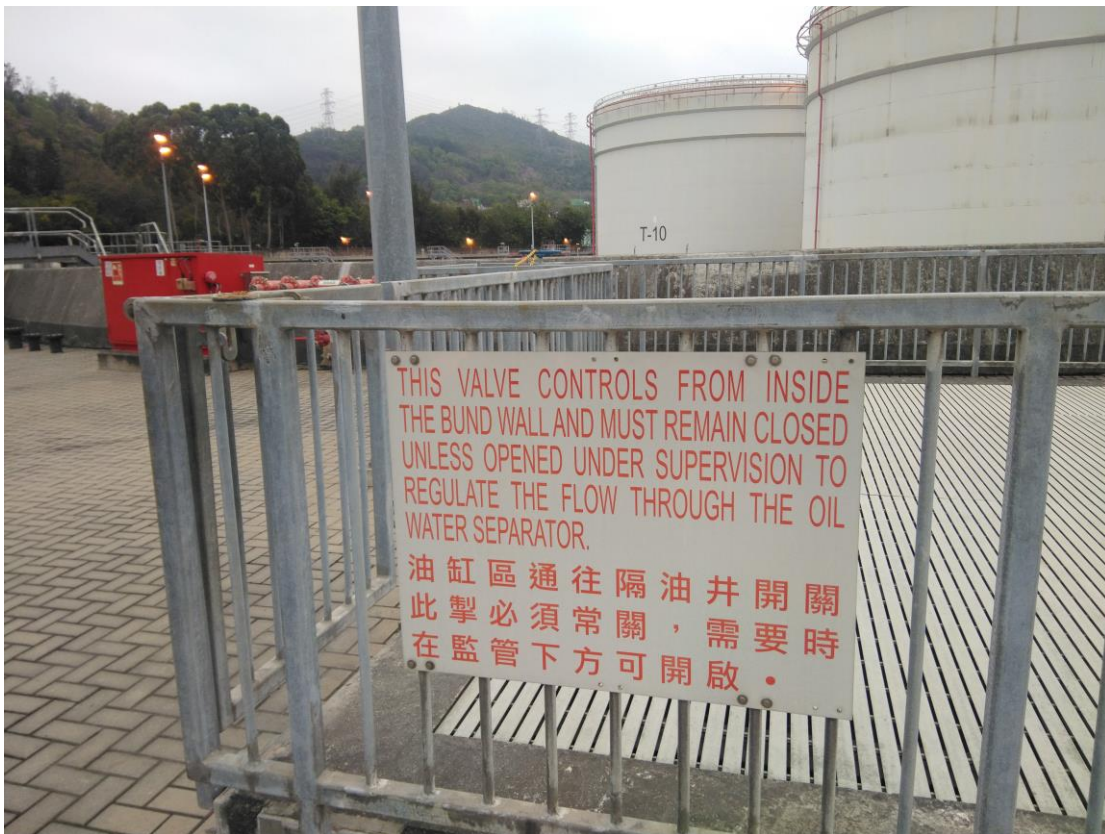
(21) Outlet valve provided for Phase 1b Interceptor with instruction sign to keep “normally closed”
