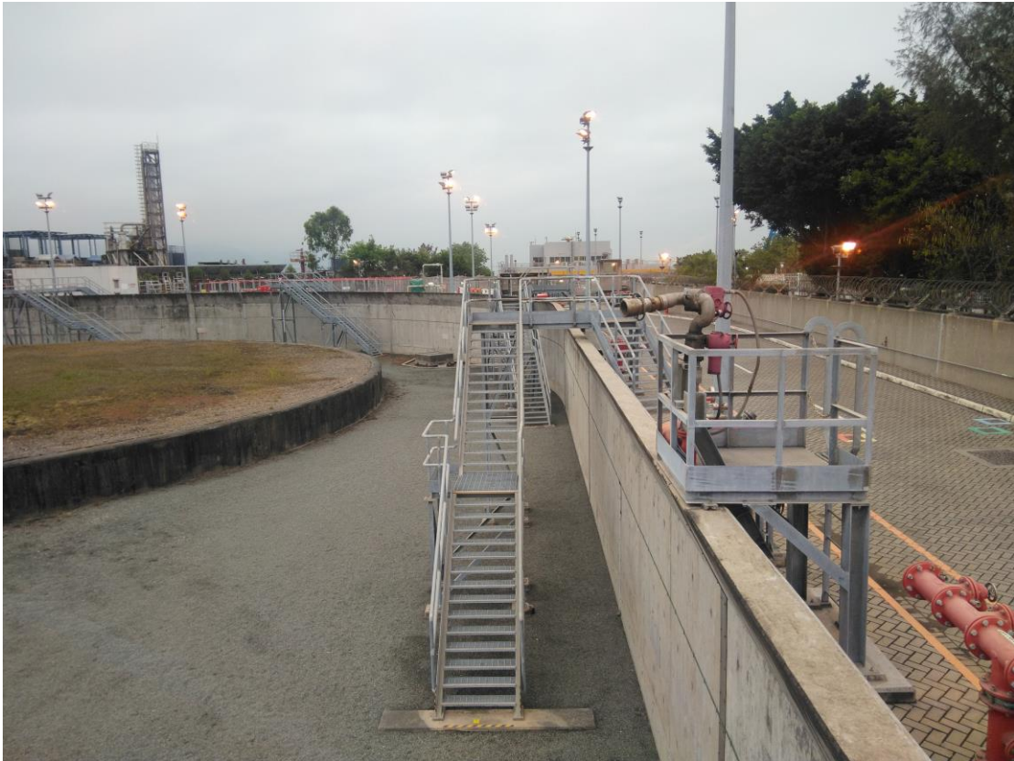
(3) Phase 1a bunded compound is lower than the ground level outside the bunds
