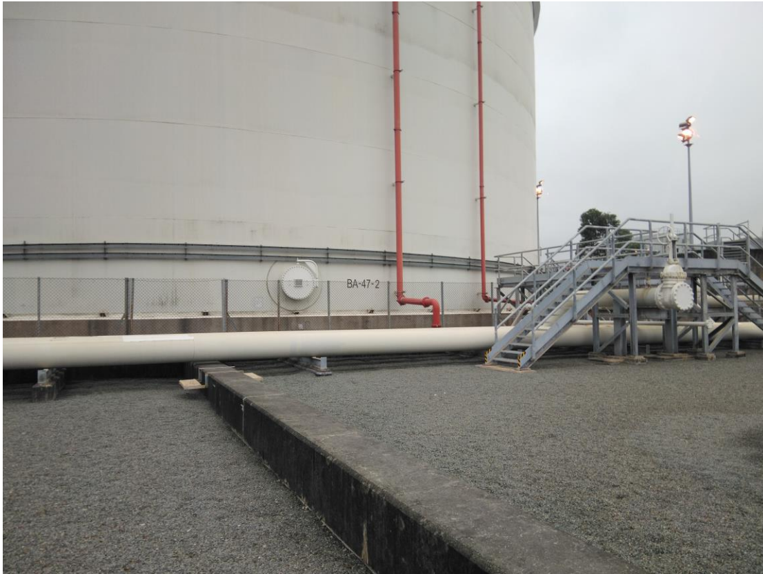
(9) Intermediate bund walls are provided in place near T-01-002
