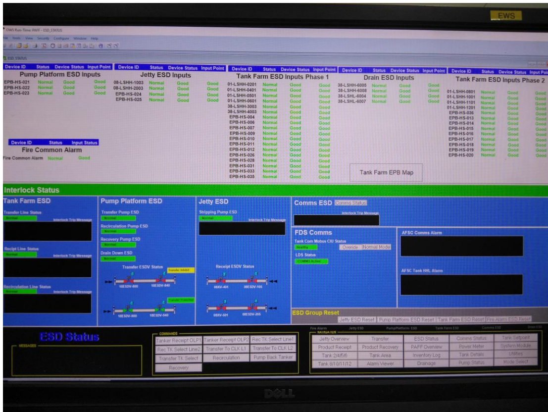
(31) The ESD regular testing as shown in SCADA System
