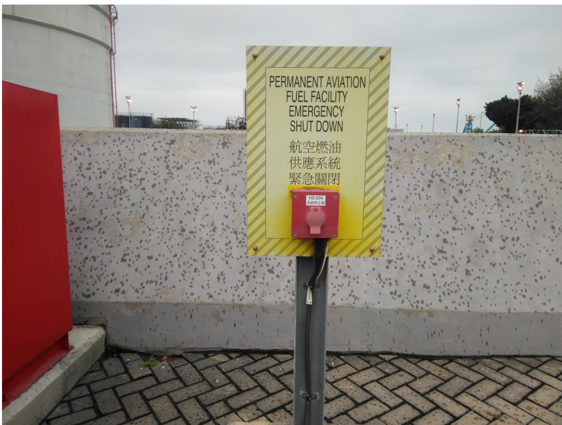
(30) ESD device is maintained in good condition and being tested periodically
