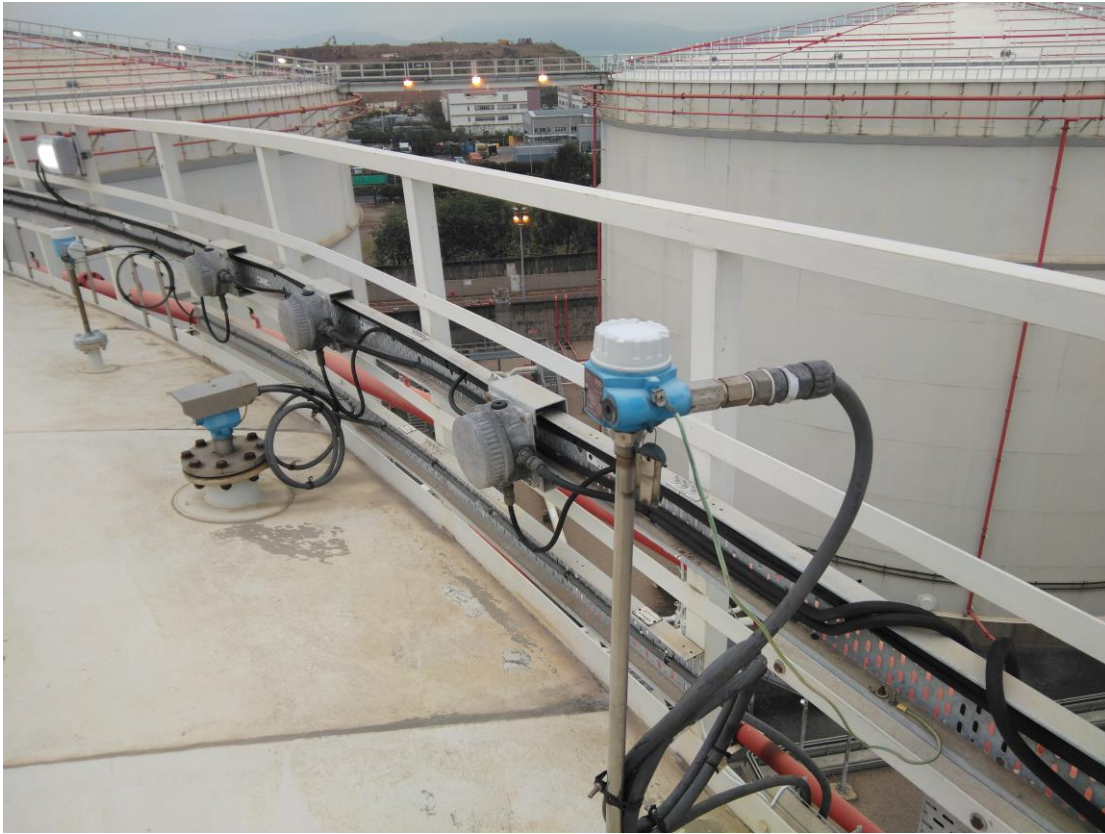
(25) Regular inspection performed on overfilling monitoring device (High-High Level Alarm)
