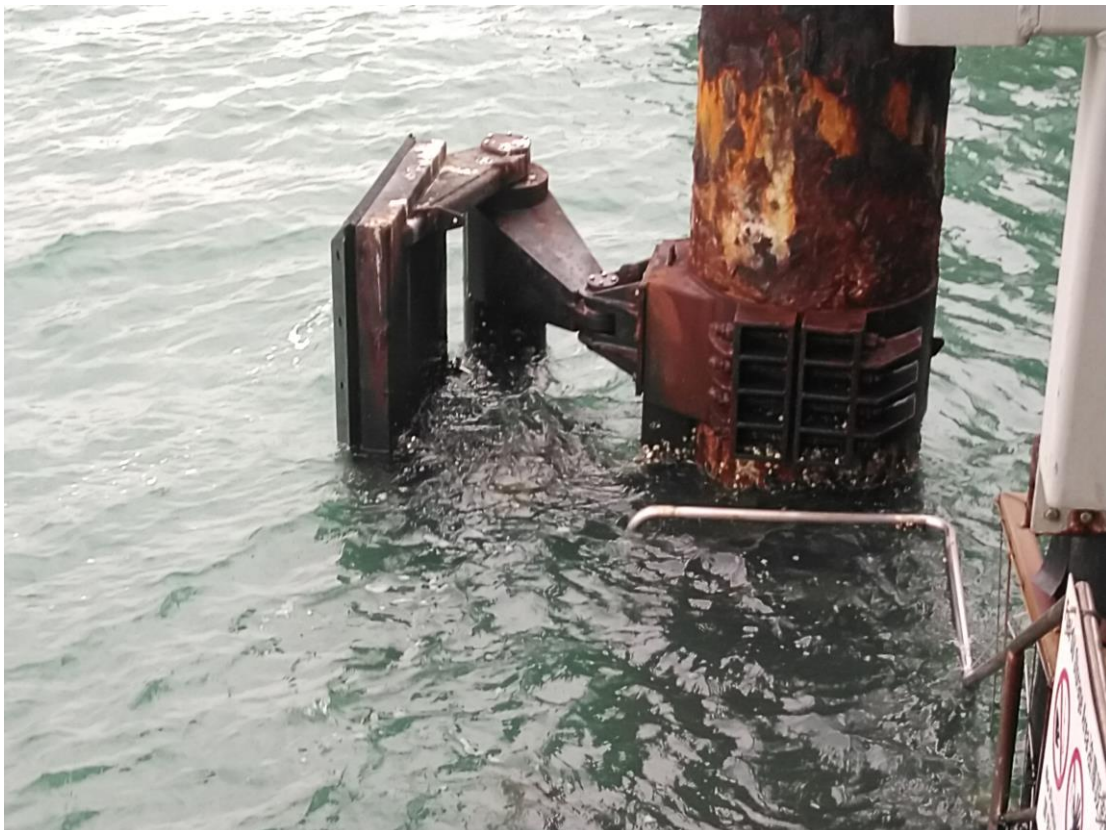
(38) Fenders are installed at shore side of the jetty
