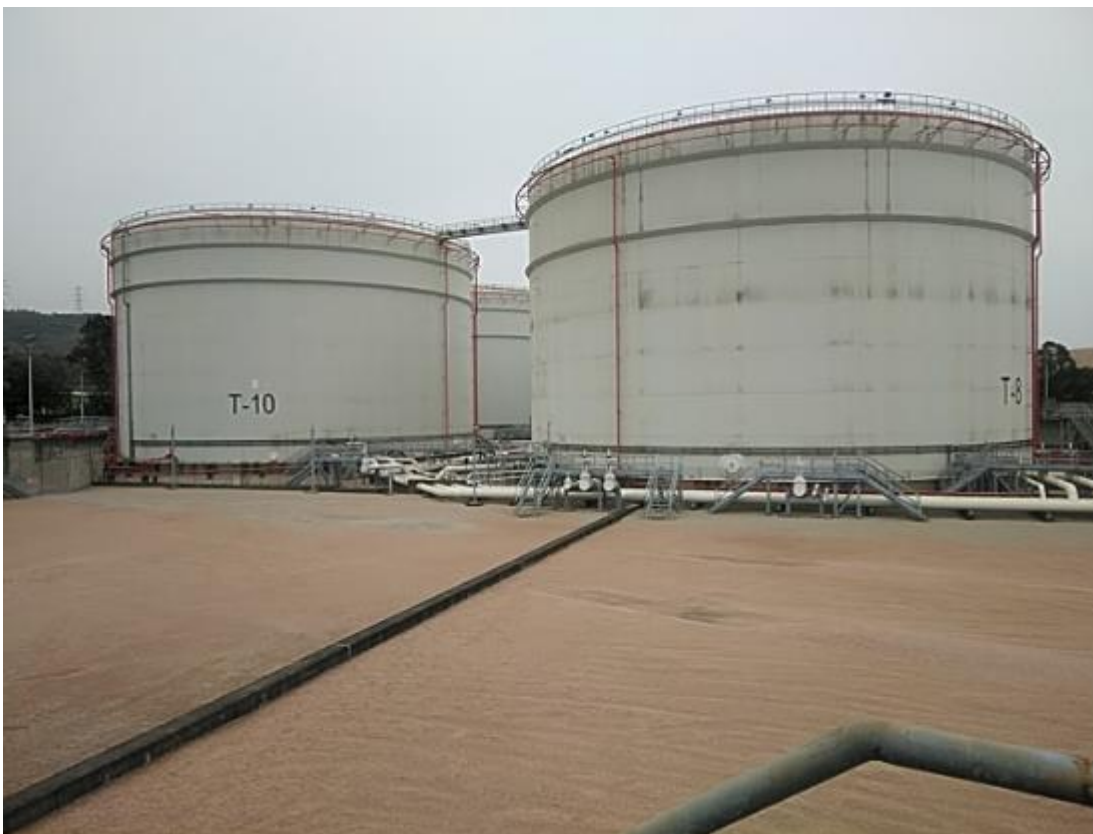
(2) Four tanks are located within bunded compound – Phase 1b
