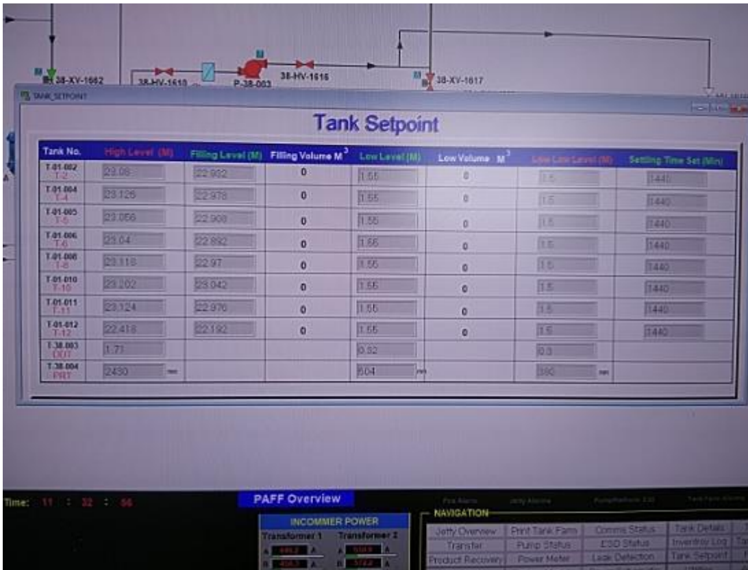
(24) High Level Alarm being set in the SCADA System
