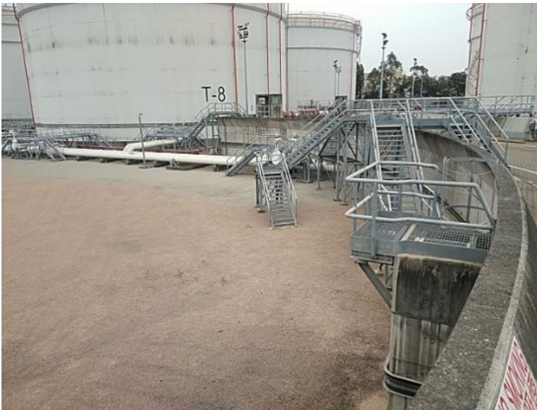
(4) Phase 1b bunded compound is lower than the ground level outside the bunds
