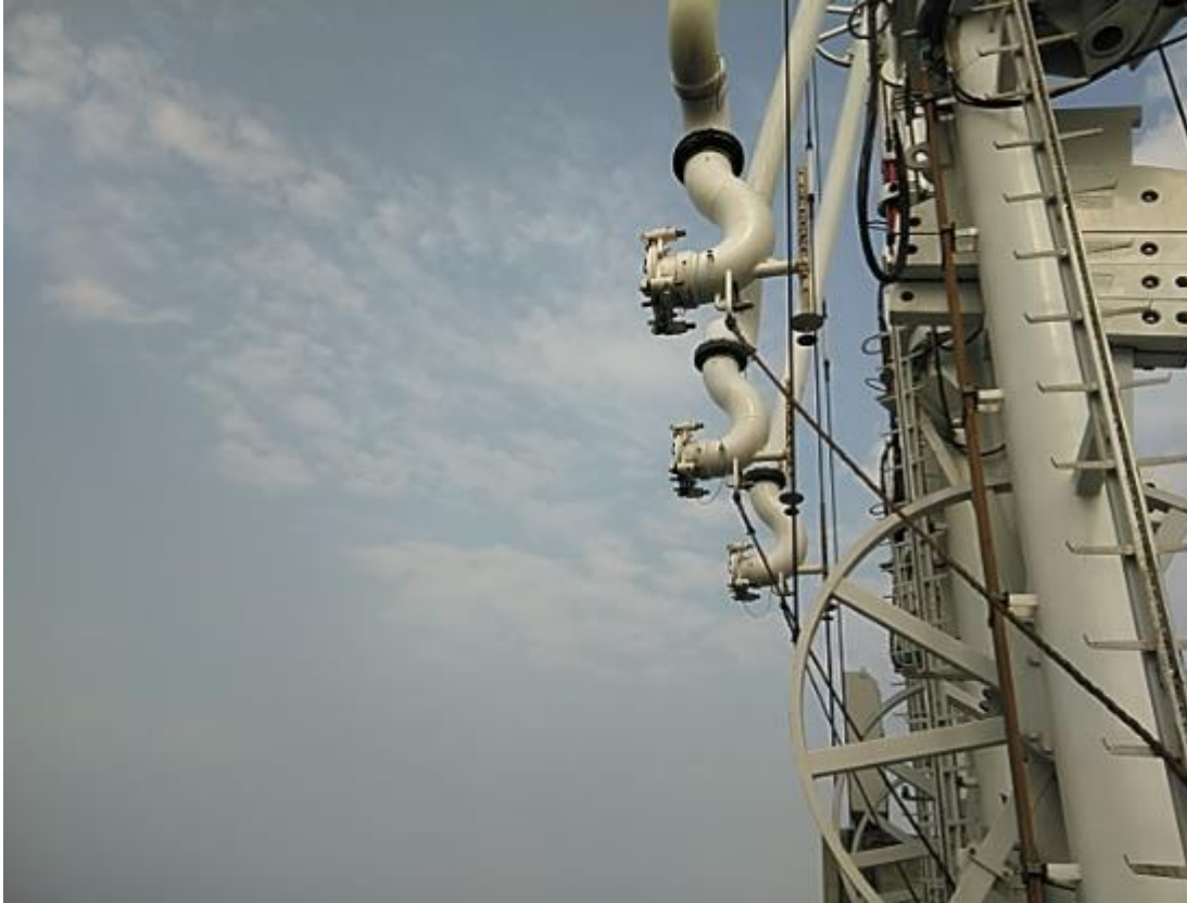
(39) Slop collection utilities are used for coupling and de-coupling of the loading arms
