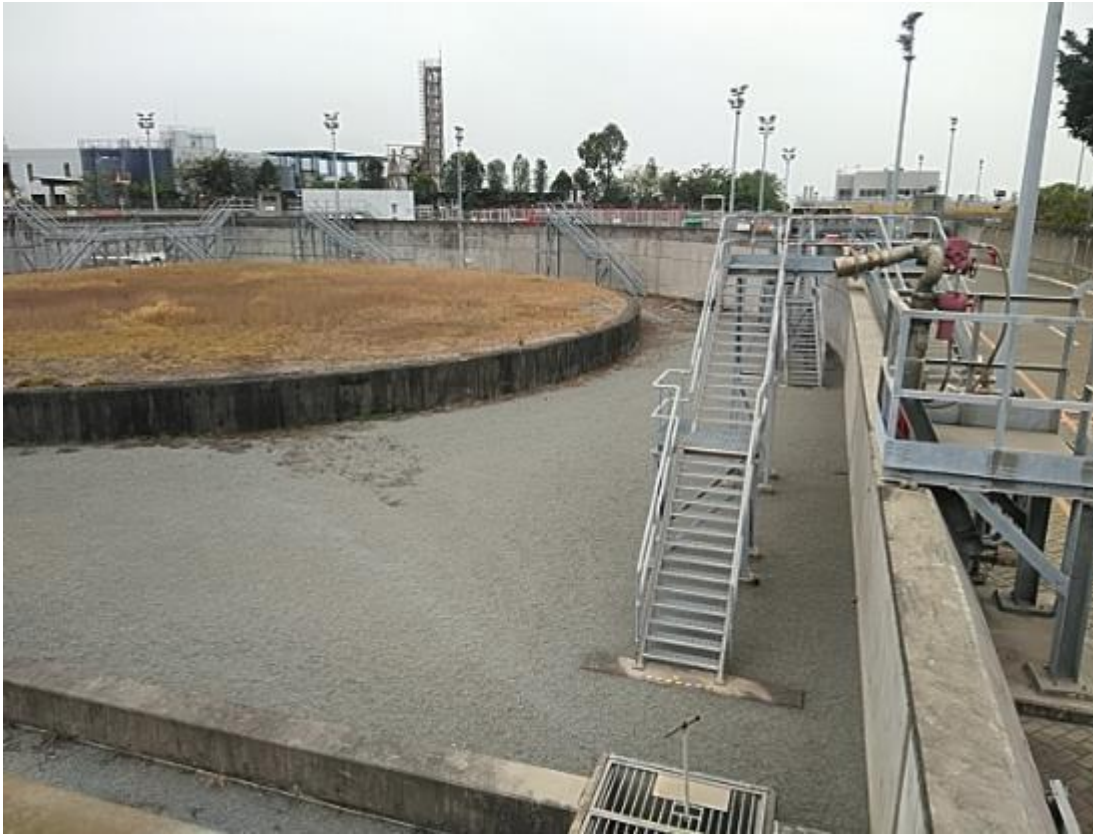
(3) Phase 1a bunded compound is lower than the ground level outside the bunds
