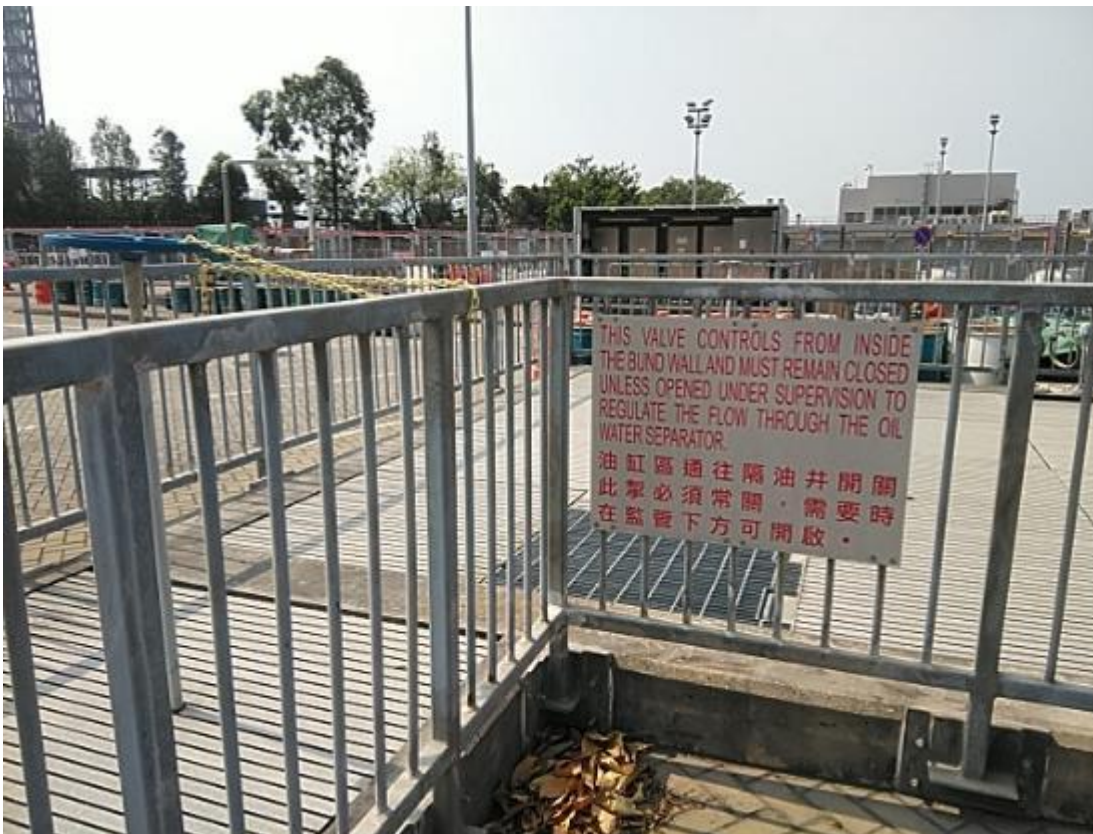
(20) Outlet valve provided for Phase 1a Interceptor with instruction sign to keep “normally closed”
