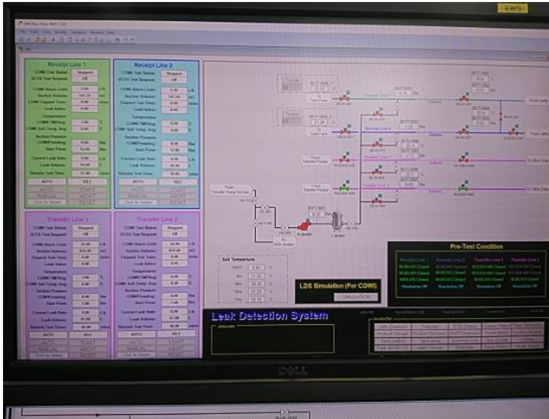
(27) Leak detection “COWI Stat Leak System” installed into computer
