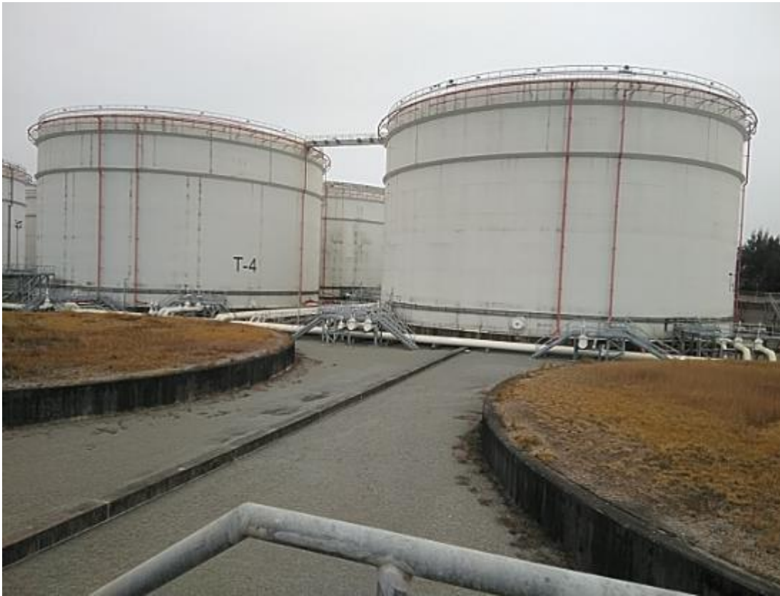
(1) Four tanks are located within bunded compound – Phase 1a
