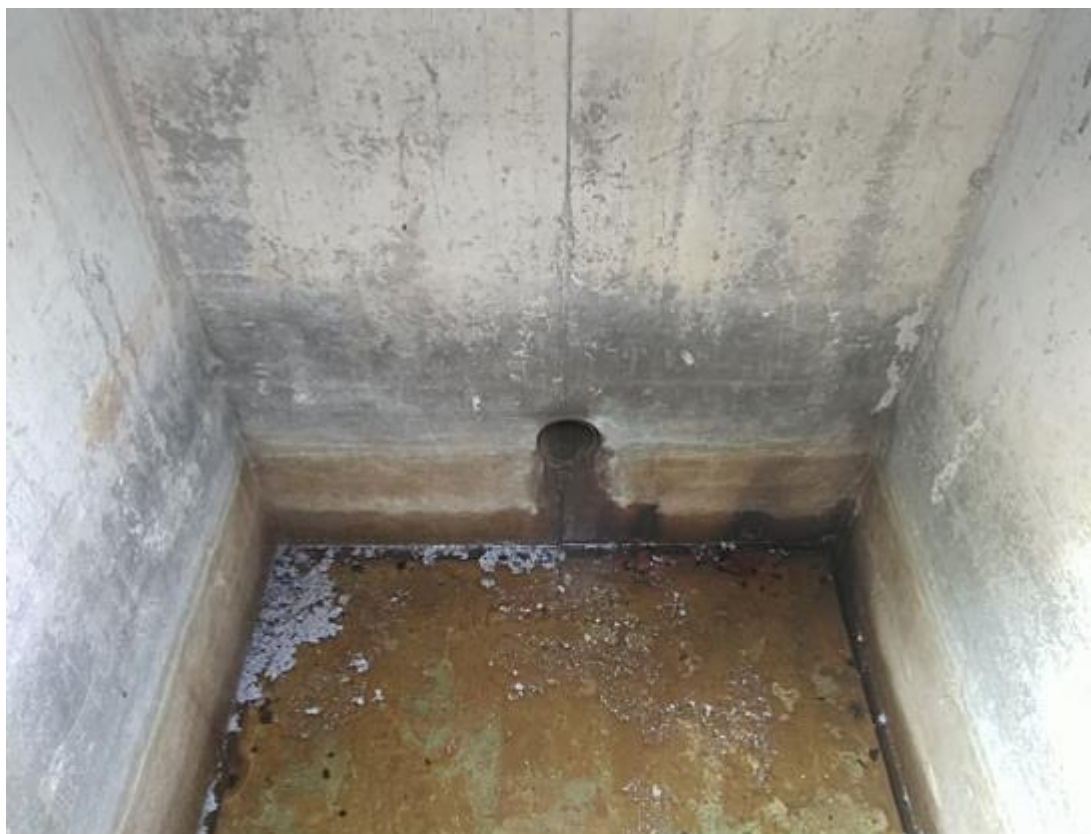
(28) Leak detection tell-tale pipe underneath the storage tank opens out to a collection chamber
