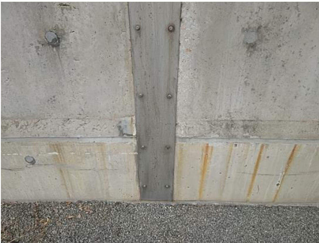
(6) Visible parts of the joints are covered by stainless steel plates on the inside at phase 1a bund
