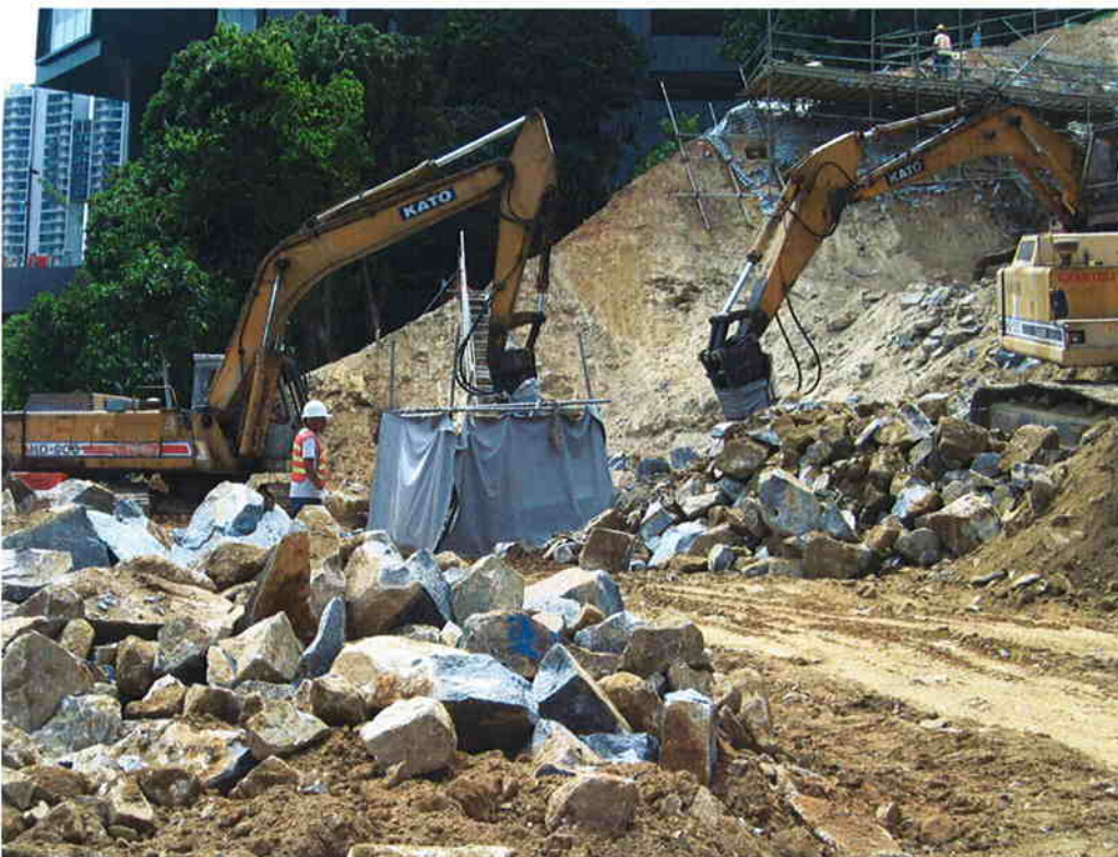
2. Sound insulation sheet surrounding the rock breaking activities as far as possible.
