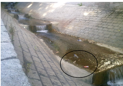
Rubbish was observed at I-1-C
