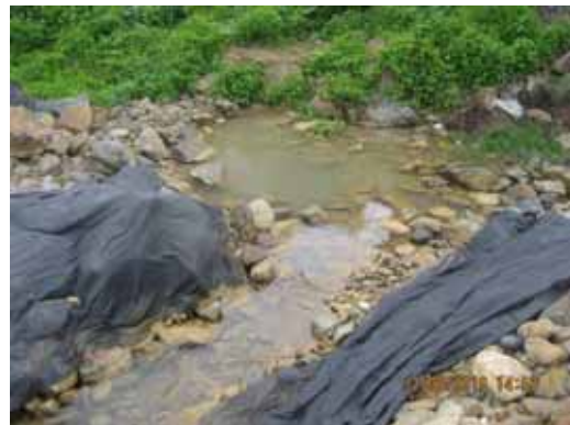
Fig.4.2 – Some of the haul access was not completely protected with proper earth bund and/or barriers
