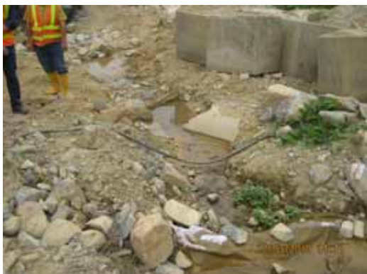
Fig.6.1 – Barriers with geo-textile coverings were provided along the site diversion channel at ch.50
