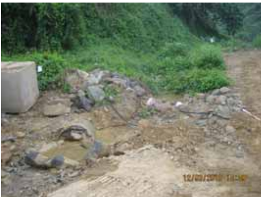
Fig.4.1 – Site water diversion channel at ch.50 was exposed without geo-textile coverings
